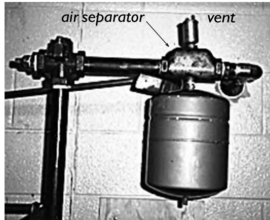
Expansion tank, air separator, and Vent:
