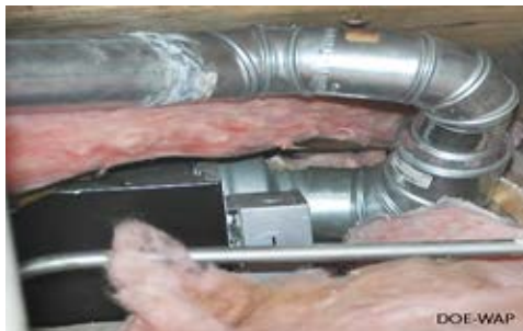
Wrong-way fan orientation: Turning the air stream 180 degrees substantially reduces airflow.
