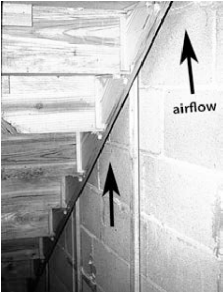
Unfinished stairways: Unfinished spaces underneath stairs create major air leakage pathways between floors and between the attic and crawl space or basement.
