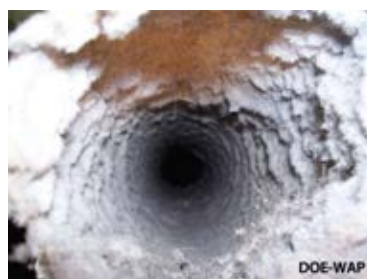
Lint collection: After years of operation, lint coats flexible pipe and eventually blocks the airway.
