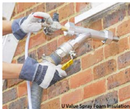
Injectable foam: Installers inject low-density foam into a cavity behind a single brick wall.
