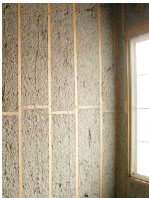
Spray fibrous insulation: Installers blow wet-spray fibrous insulation into cavities and shave off the excess.
