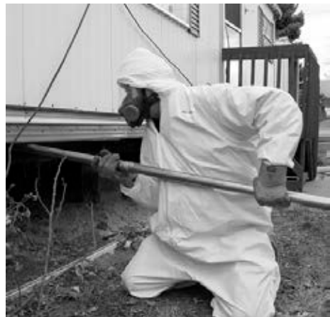
Patching a flexible belly: The technicians uses both adhesive and stitch staples to fasten a patch.
