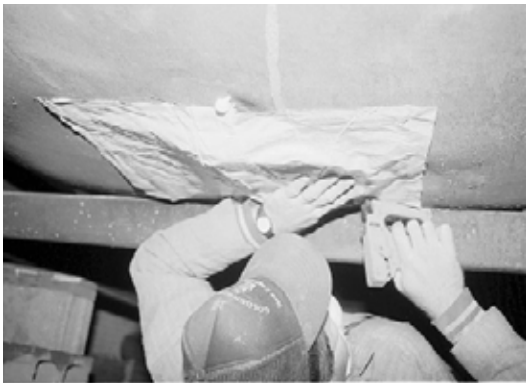
Blowing a floor through the belly: The contractor inserts a rigid fill-tube through the belly to blow insulation into the floor cavity and underbelly.
