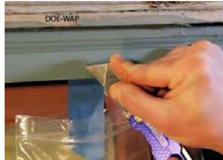
Cut through all the layers of paint. Also install a bag beneath the cut to catch paint fragments.
