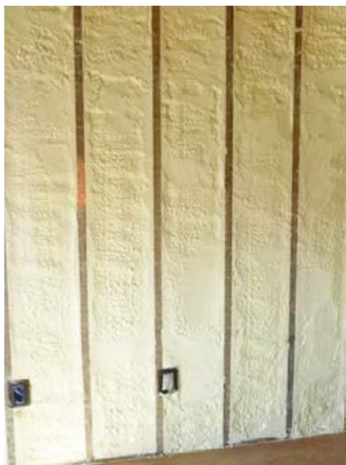
Sprayed closed-cell foam: Installers spray closed-cell foam short of filling the cavity or else they shave the excess off.
