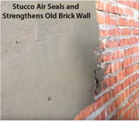
Stucco over brick: This retrofit serves two purposes: air sealing and structural reinforcement.
