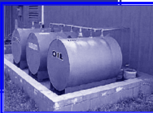
Aboveground tank storage of vehicle fluids.
