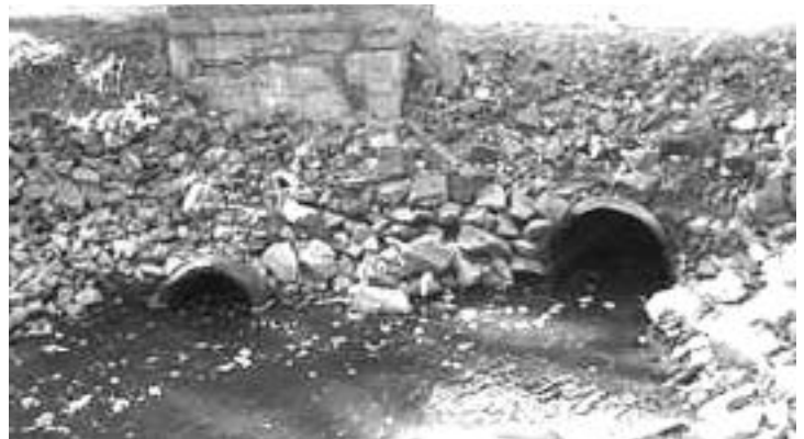
A new culvert (right) allows increased tidal flushing of Mill Meadows wetland.
