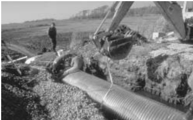
DEP staff installing an aluminum culvert in a dike at Impoundment IV at the Barn Island Wildlife Management Area, Stonington, to restore tidal flow.
