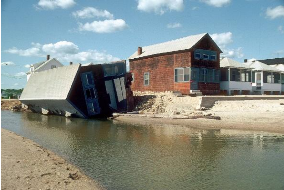
Figure 1: The foundation of this house in Lyme was destroyed by water escaping from an inland marsh serviced by undersized culverts
