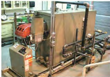
PHOTO A. A B100-fired boiler in a Brookhaven National Laboratory test facility.
