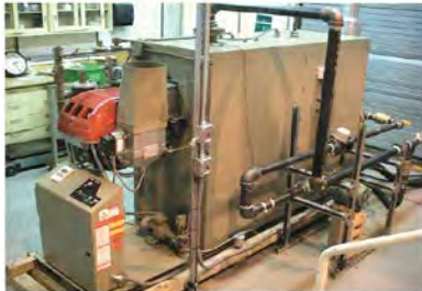
PHOTO A. A B100-fired boiler in a Brookhaven National Laboratory testing facility.
