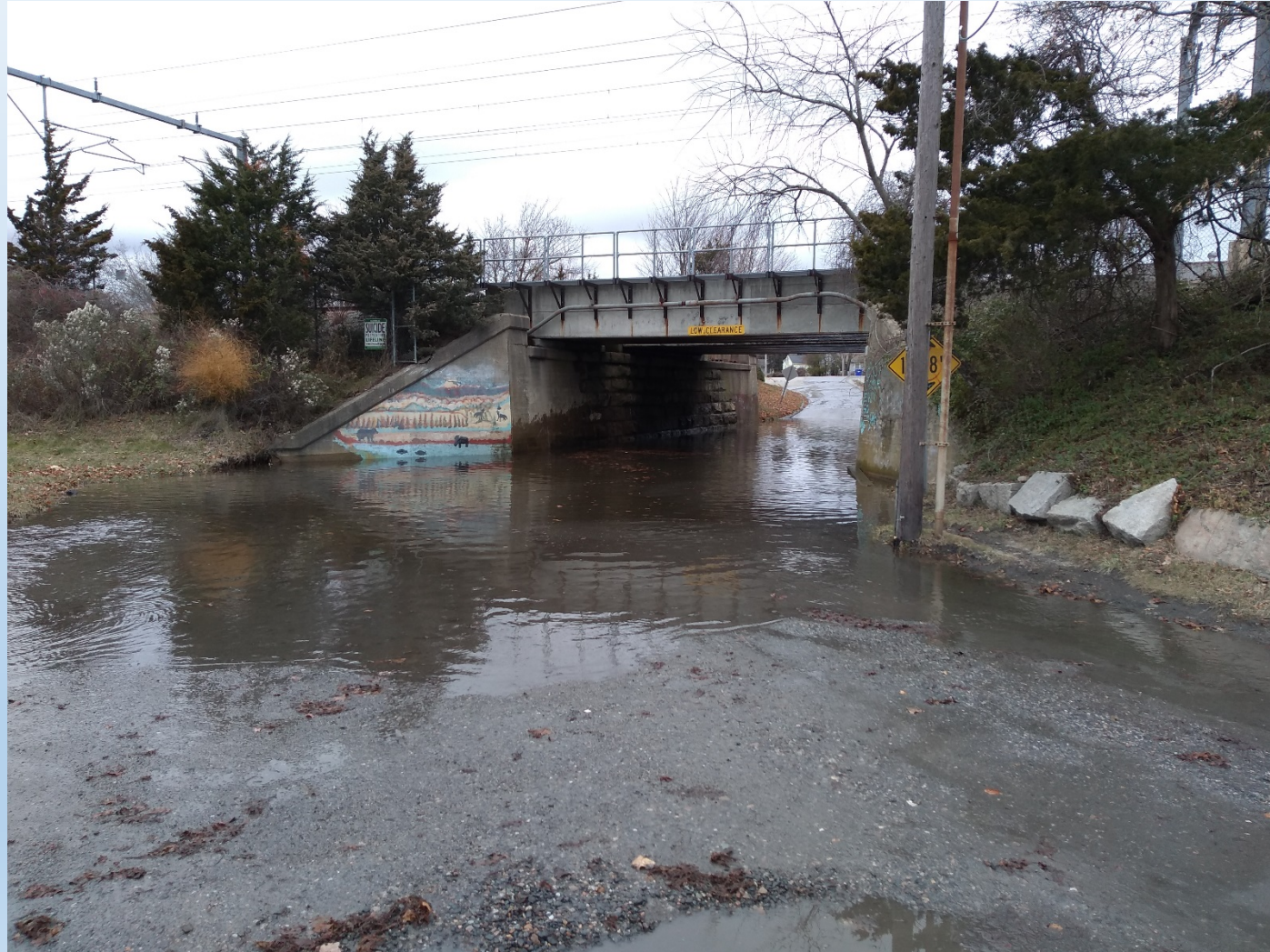
2 feet of tidal water at Amtrak overpass from catch basin surcharge/Poquonnuck River flooding
