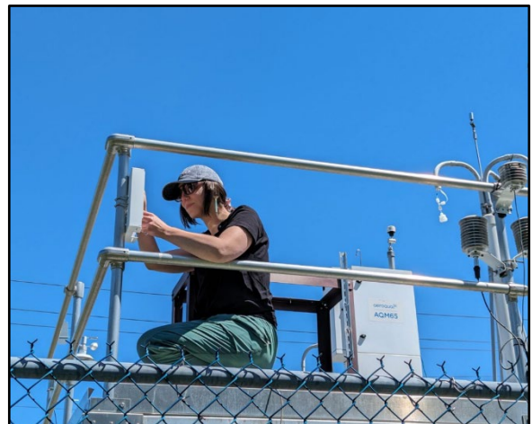
Right: Installation of low-cost air sensor used in collocation studies at East Hartford monitoring site
