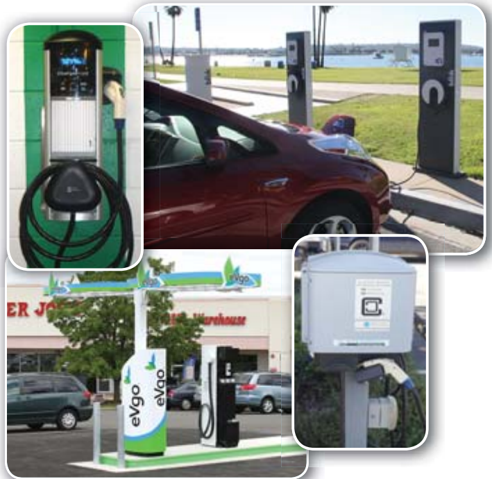
Level 2 charging stations from different manufacturers.
