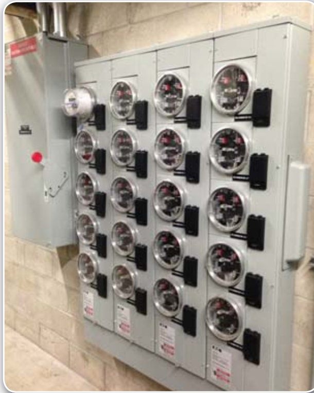
EVSE-specific meters in a MuD meter room.
