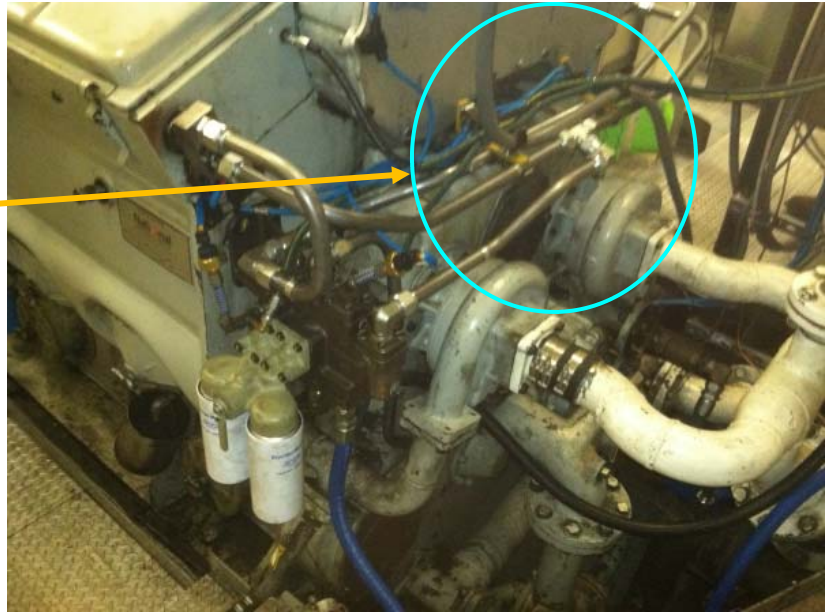
Mechanical Governor Removed (circled in Blue)
