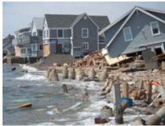
Structure removed from pilings at Cosey Beach, East Haven View Larger Image
