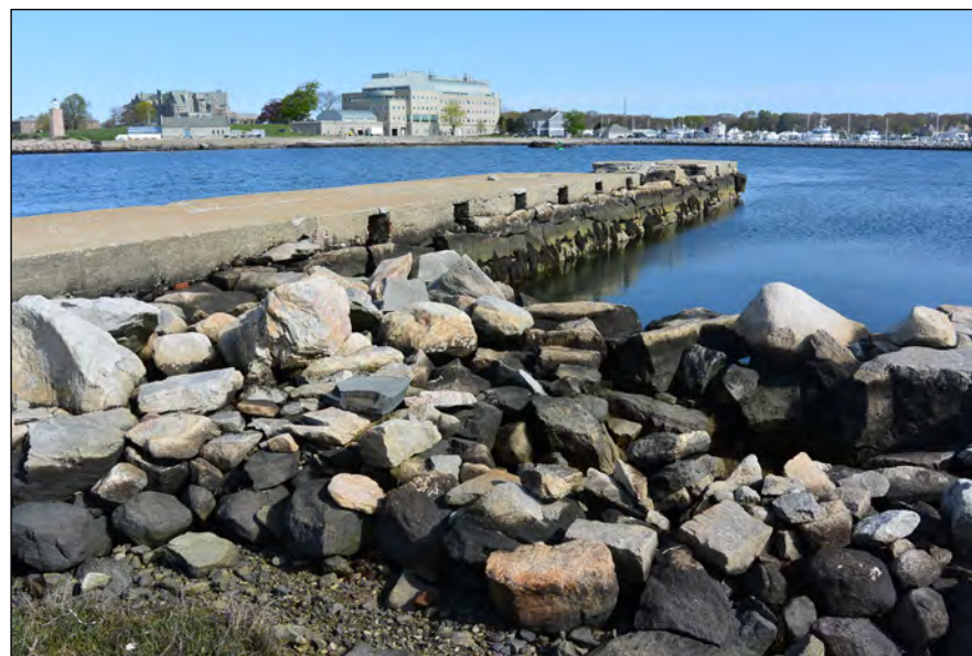
Photograph showing the stone wharf with concrete cap at Pine Island (Photo by R. Christopher Goodwin & Associates)
