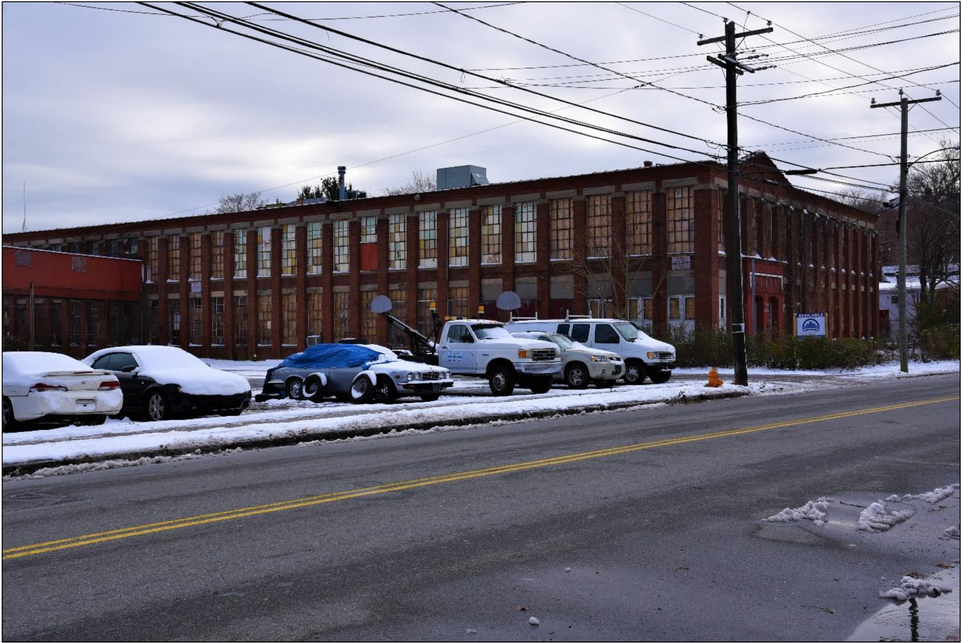
North and eastern elevations of Building No. 1. (1919), camera facing southwest. Photograph 1 of 27
