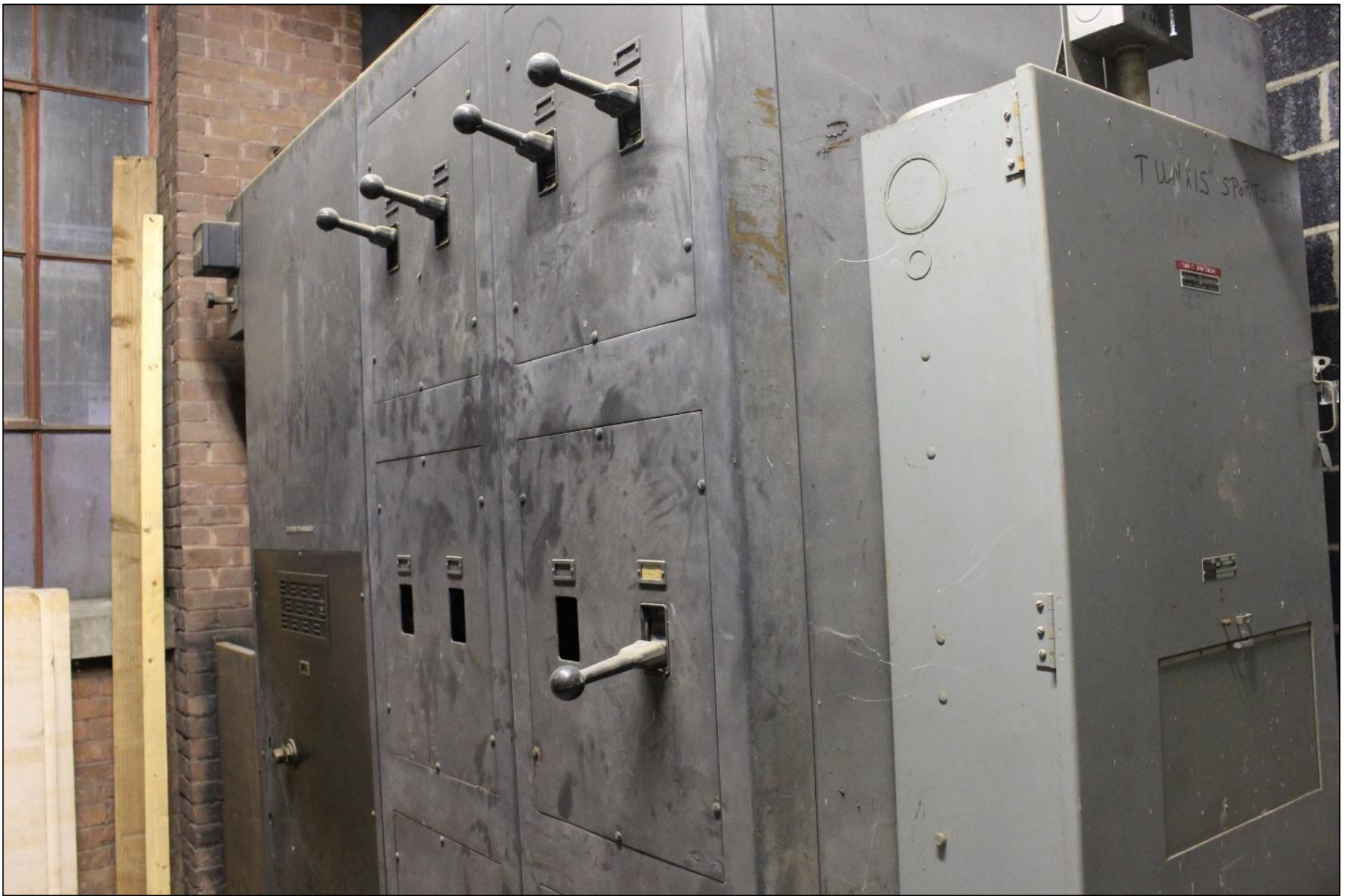
Electrical Panels in Building No 2. (1919)
