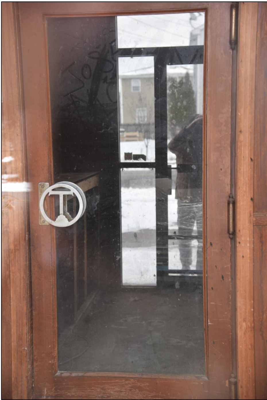
Vestibule in Building No.1 ell (1919), first floor, camera facing south. Photograph 14 of 27
