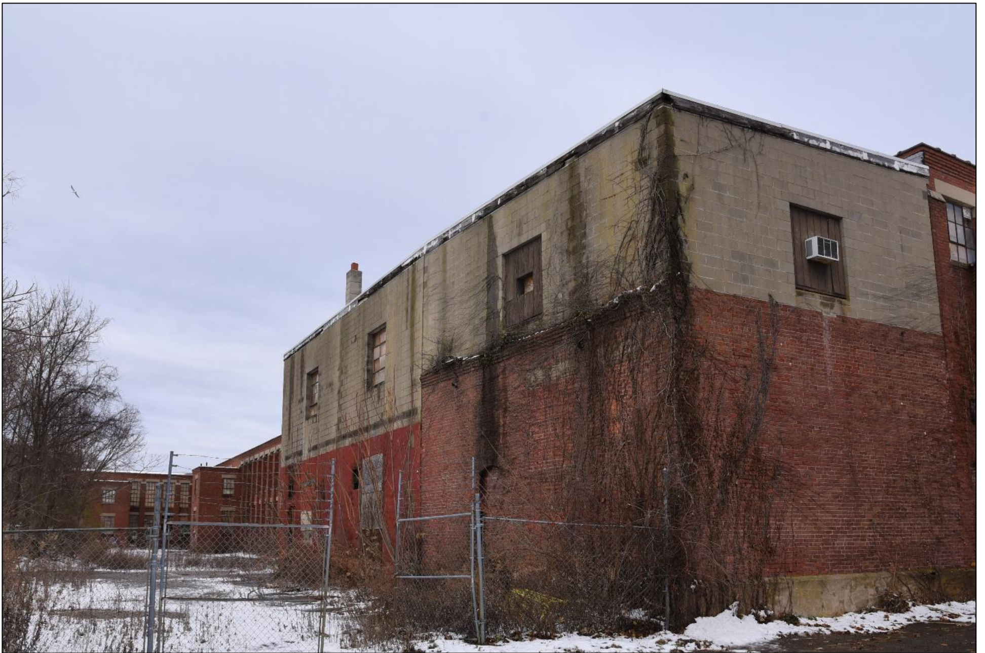
South and west elevations of addition (ca.1920-1960), camera facing northeast. Photograph 6 of 27
