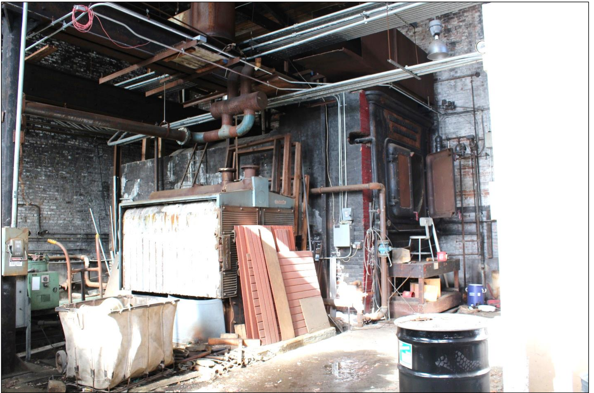
Interior of Building No.2 (1919) with Bigelow boiler, camera facing northeast. Photograph 18 of 27
