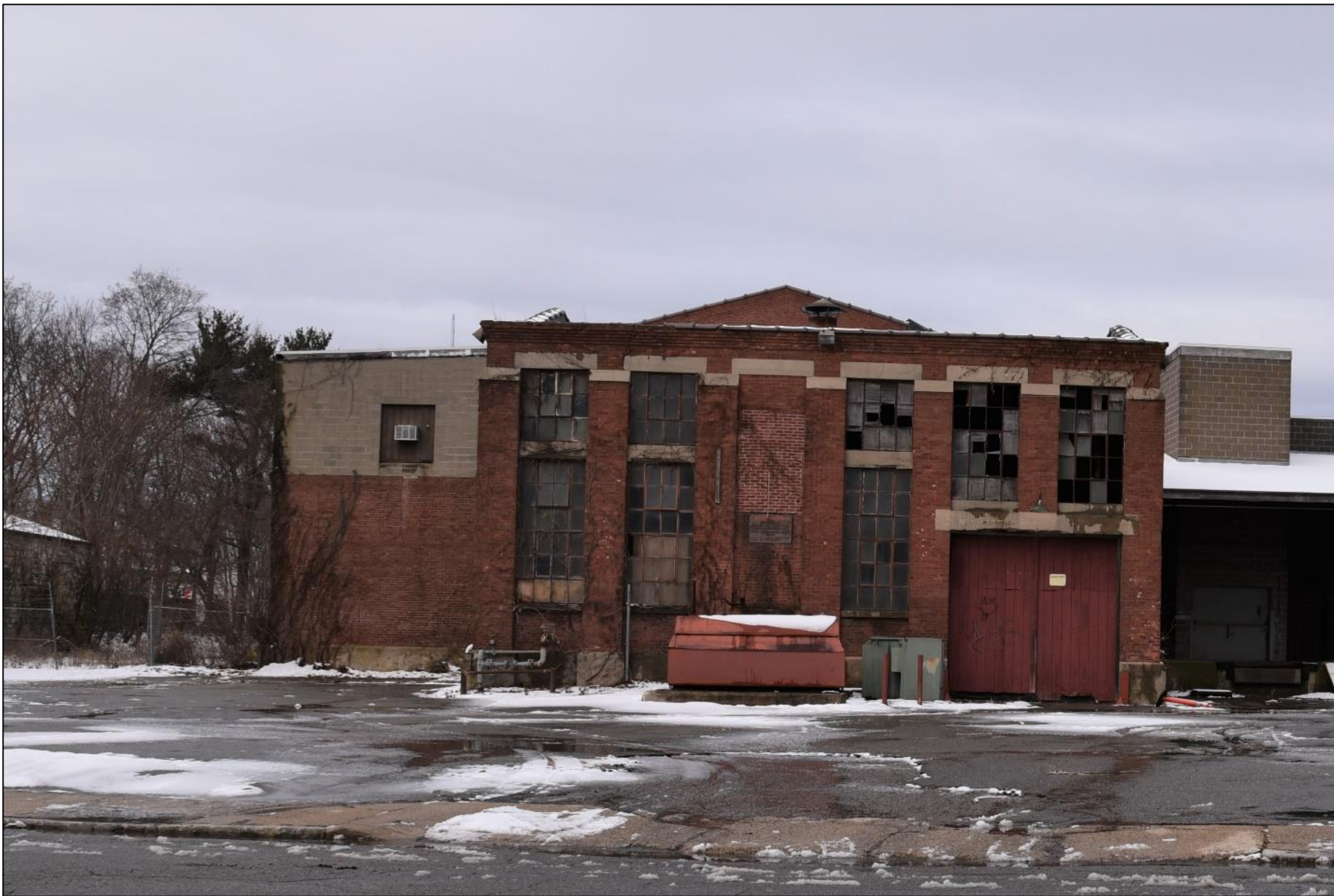
Southern Elevation of Building No. 1 (1919) (obscured by boiler house (1919), camera facing north. Photograph 5 of 27
