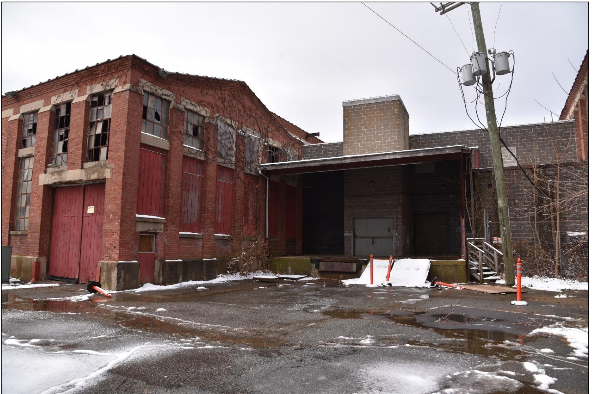
Southern and eastern elevations of Building No. 2 (1919), left, and southern elevation of loading dock and elevator shaft (ca.1960), camera facing northeast. Photograph 17 of 27
