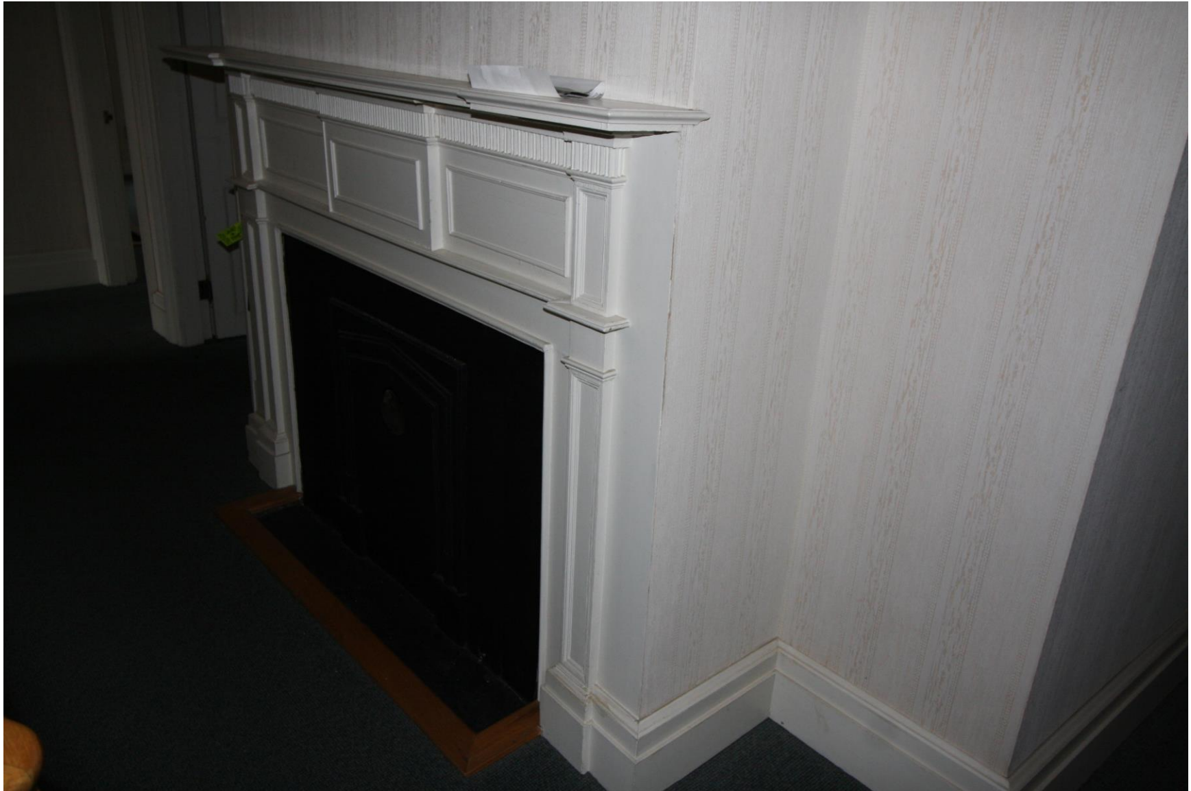
Photograph 13A. Interior elevation, west wall central second story southern room. This room is now the location of the new central stairs.
