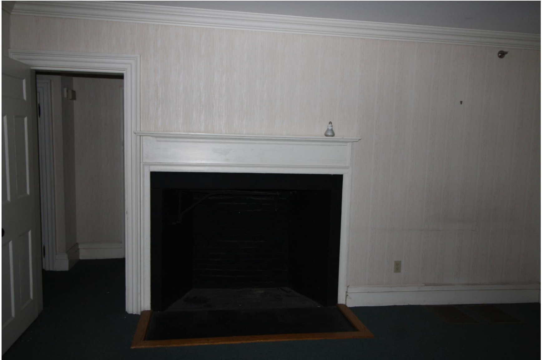
Photograph 7A. Fireplace in southeasternmost room of original portion of building, first floor (original kitchen north wall).
