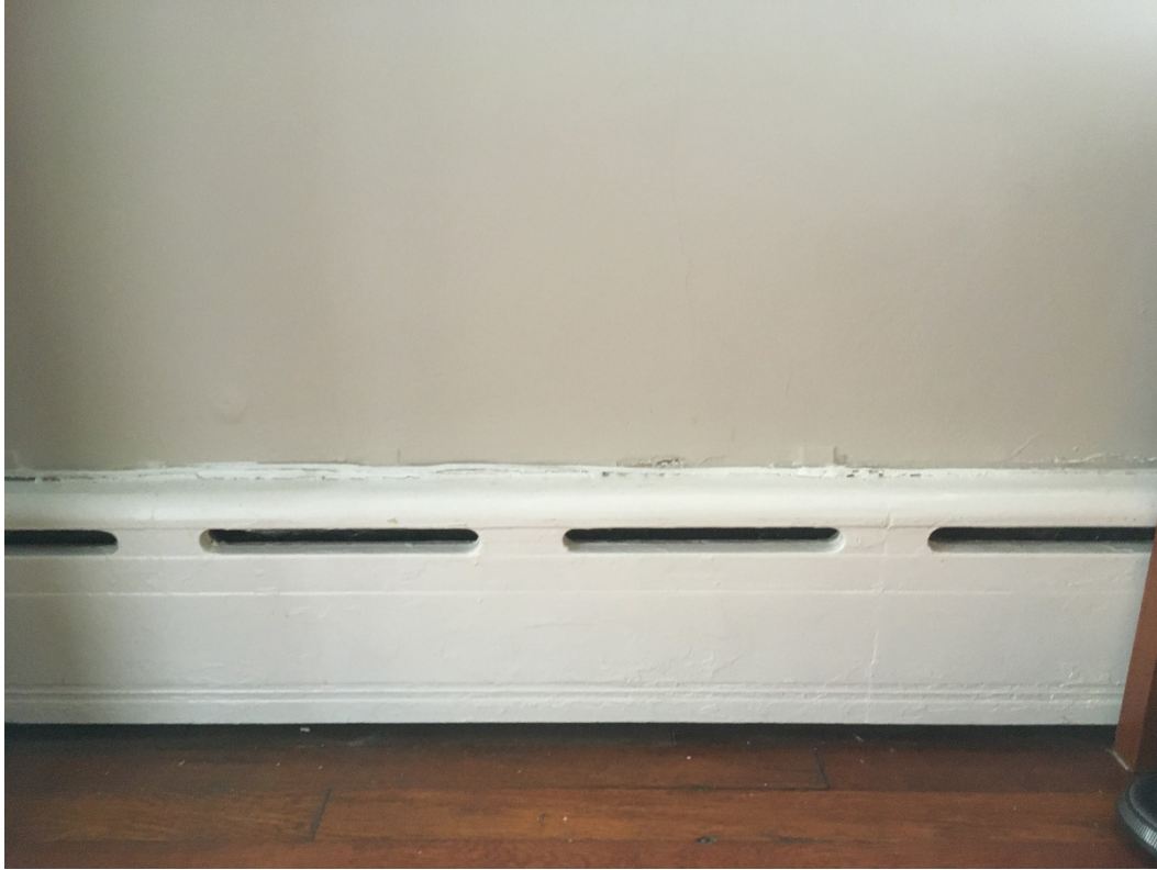
Detail of baseboard heat vent, 12/2/20.
