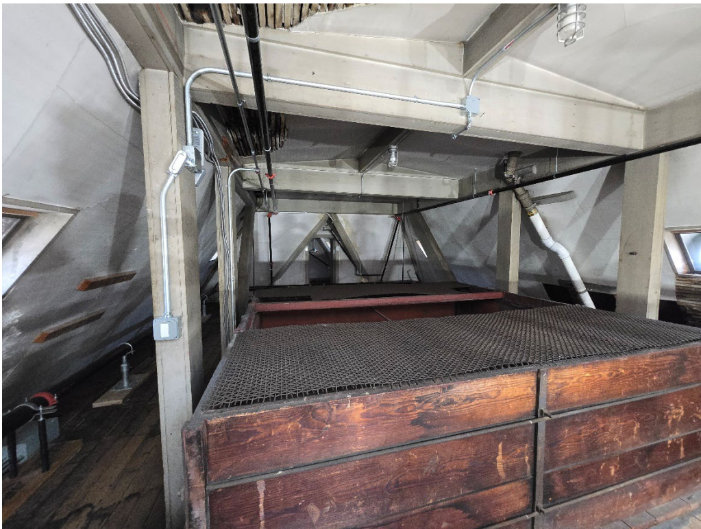
Photograph 63. Cistern in attic, view east.
