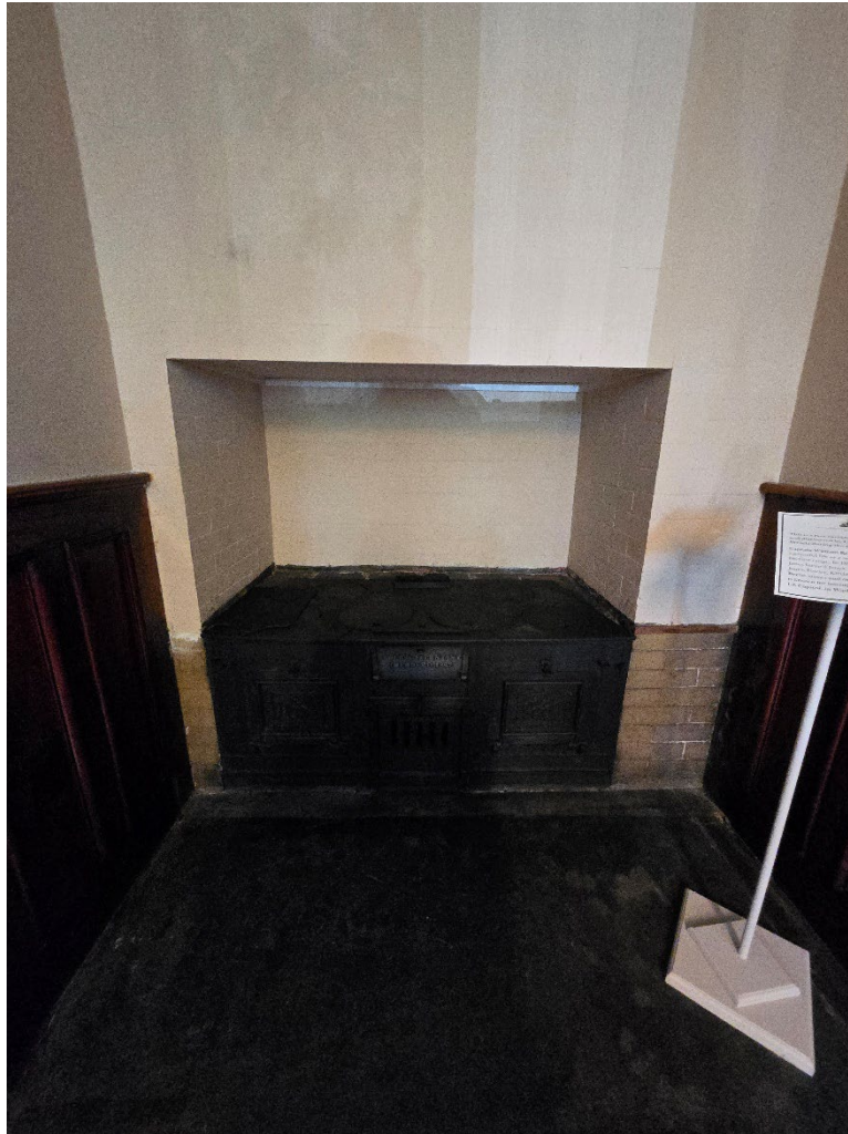
Photograph 21. Stove in Servants' dining area, view west.
