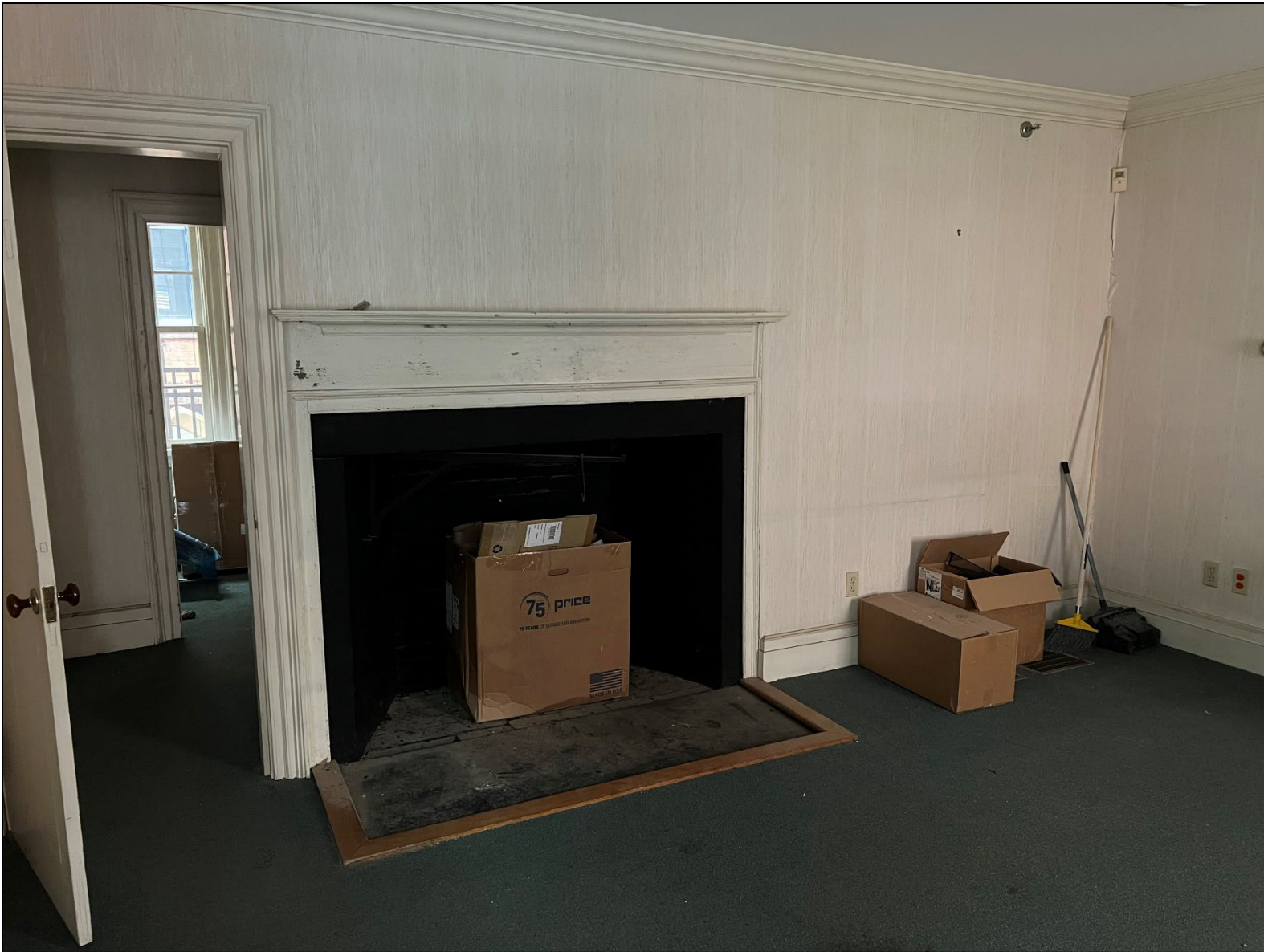
Photograph 10. Fireplace in southeasternmost room of original portion of building, first floor (original kitchen north wall), camera facing north.
