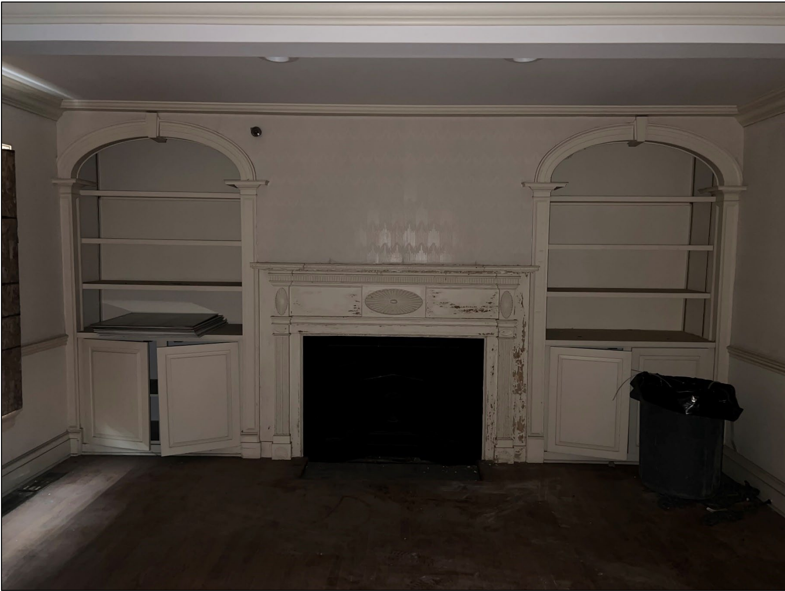
Photograph 7. Interior elevation of north wall, first story front room, camera facing north.
