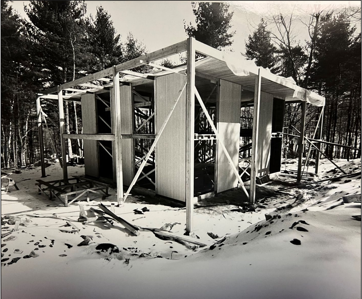
Figure 8. The System House during construction (Collections of the New Canaan Historical Society).
