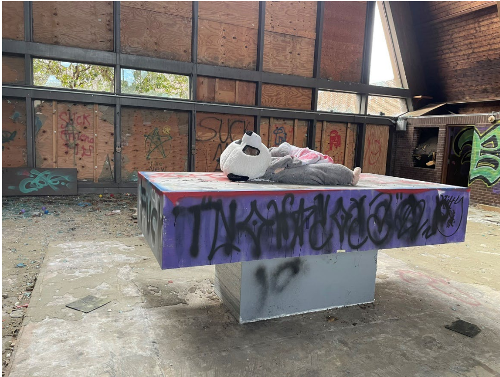
Photograph 13. Marble altar which remains in place, but is heavily damaged, view west.
