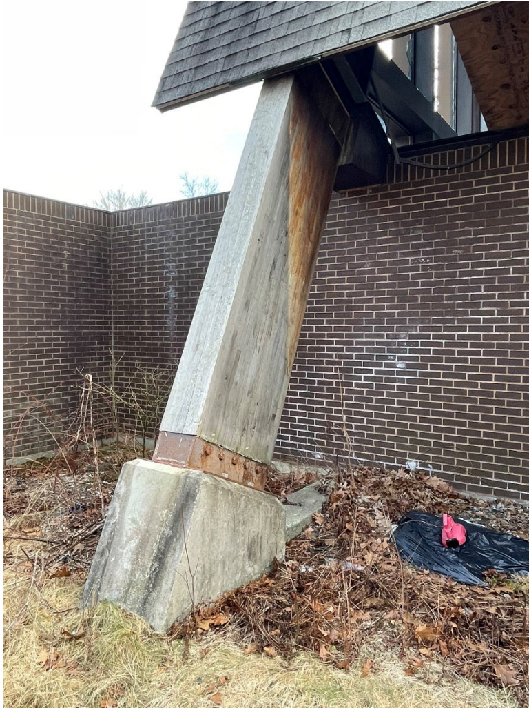
Photograph 4. Detail of concrete footing at the base of each arch, view southeast.
