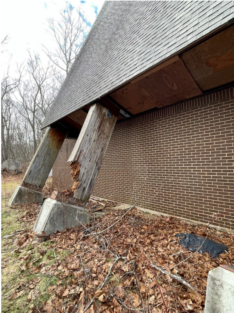
Photograph 9. Deteriorated base of an arch on the southwest corner of the building, view northwest.
