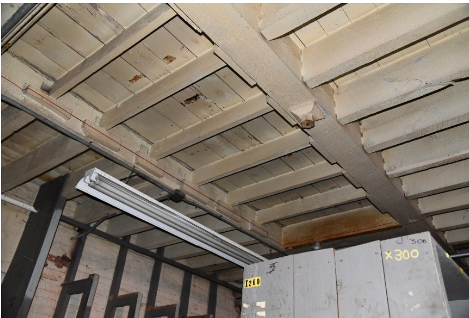
Photograph 93. Floor framing for woodworking room with double tenon joints and closely spaced joists.
