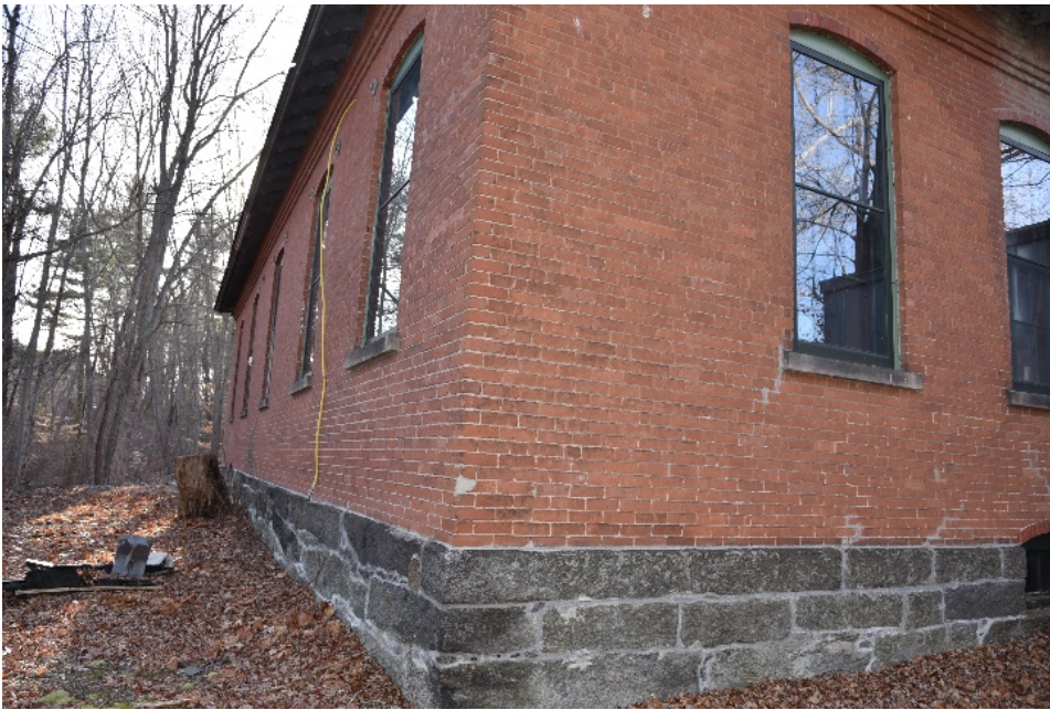
Photograph 67. East/rear and part of south elevation showing granite block foundation; camera facing south. Ground slopes down behind building.
