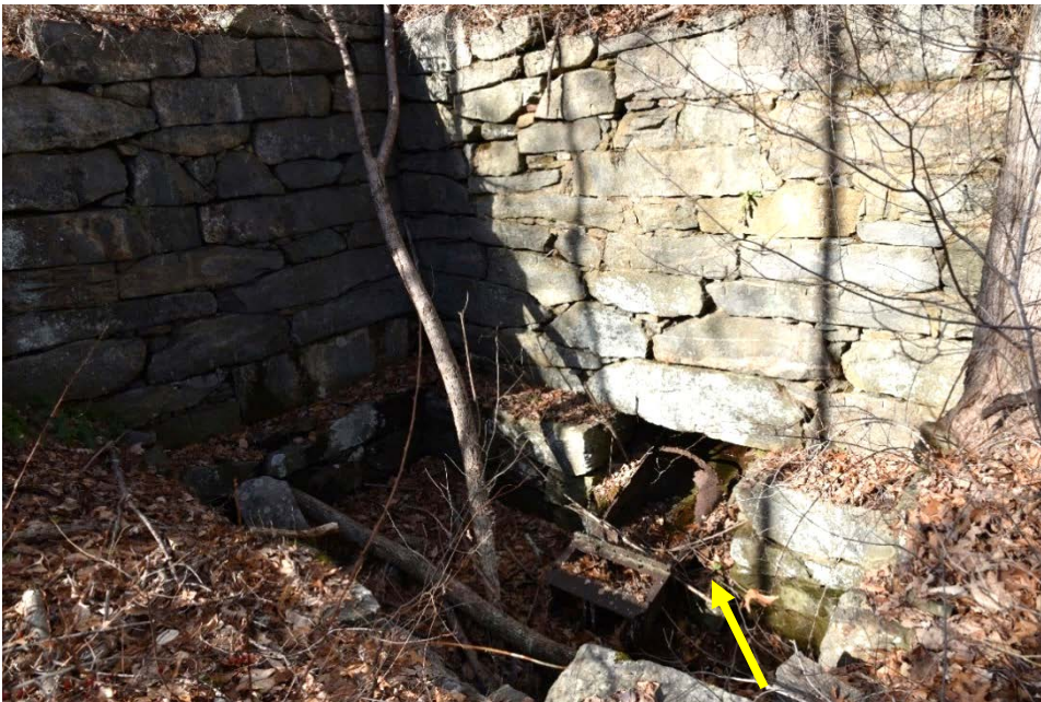
Photograph 7. Flume exiting south wall of north/south forge shop, with a metal diverter possibly allowing water to power a shaft to the east/west forge shop and iron cutting building beyond, or back to the brook; camera facing north/northwest.
