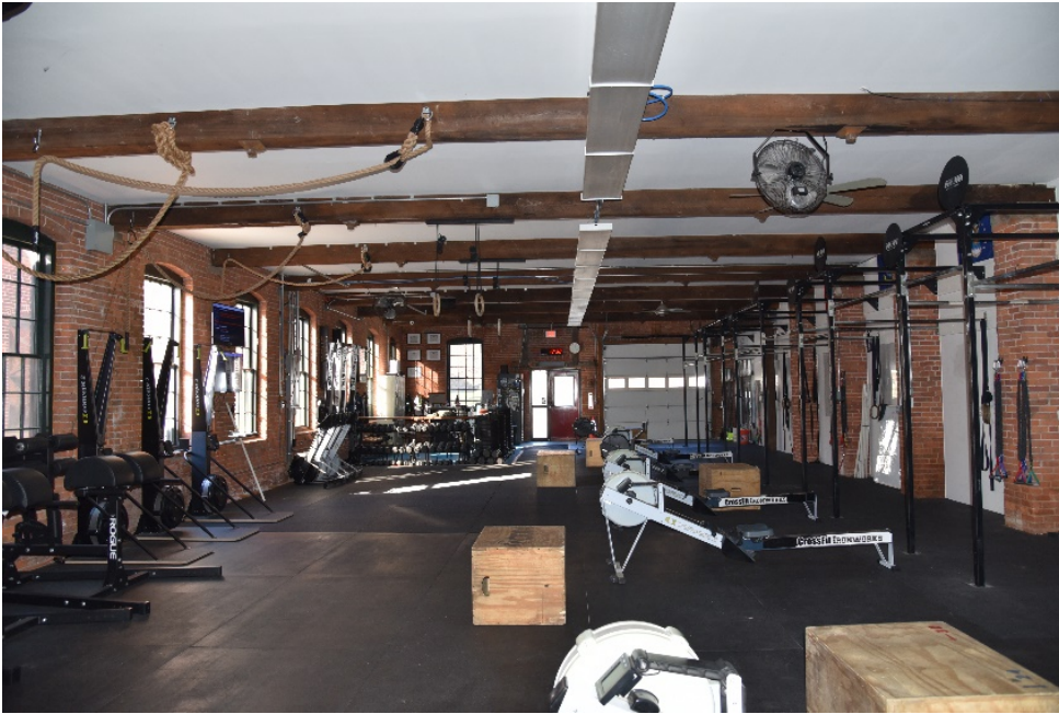
Photograph 60. Western side of ground floor of grinding/forge room; camera facing north. Timber frame sits on stones sets in brick bearing wall. Brick columns run down the center of the ground floor to carry the framing load above; non-structural walls between columns separate the eastern half of the space.
