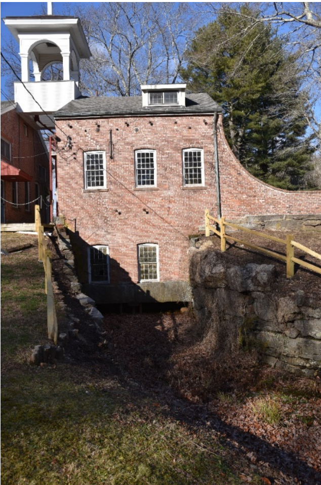
Photograph 20. South elevation of extant section of east block. Note massive sill, comprised of two pieces of granite, that supports the south wall above the tail race, and the granite walls of tail race channel.
