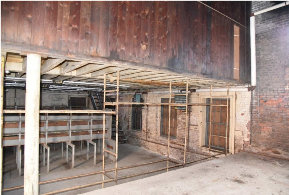
Photograph 92. Ground floor machine room open to engine room and enclosed woodworking room above.
