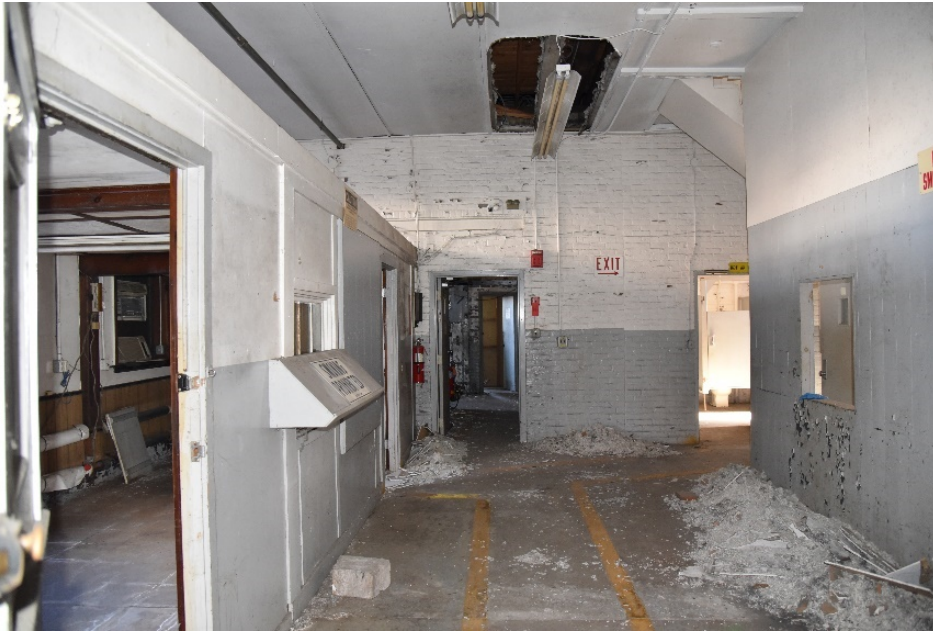
Photograph 101. Brick firewall separating office space from workspace and non-structural partition walls in eastern end of building; camera facing east.
