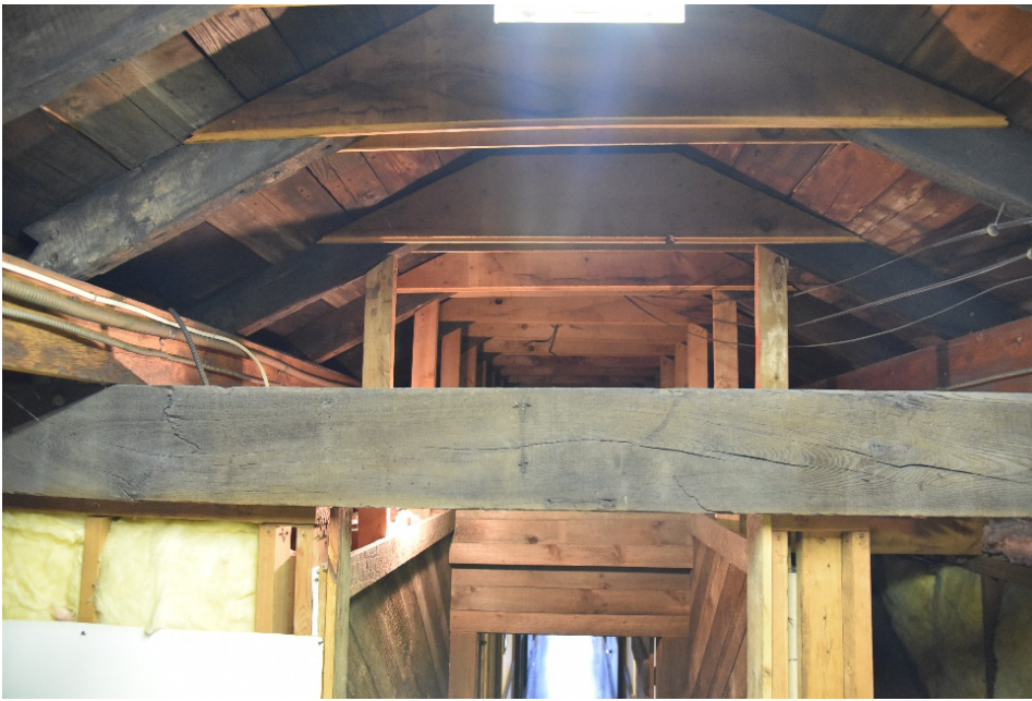
Photograph 23. Newer framing in attic corresponding to removal of clerestory and refinishing as gable roof.
