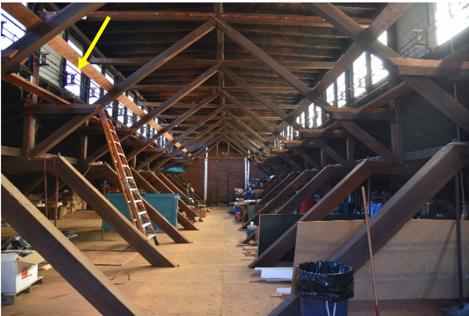
Photograph 61. Grinding/forge room, upper level, looking toward south wall. Note hardware for opening clerestory windows for venting.
