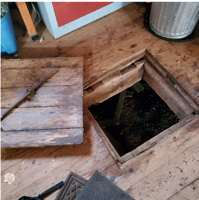
Photograph 29. Hatch to turbine chamber.
