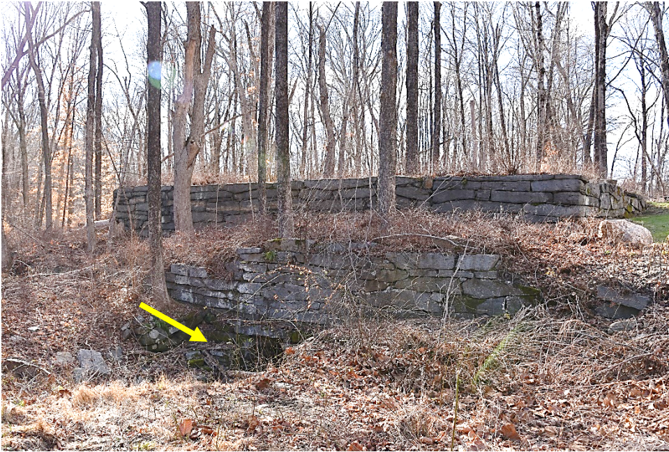
Photograph 4. Granite foundation of north/south forge shop; camera facing west toward canal. Flume pipe returns water to the brook.
