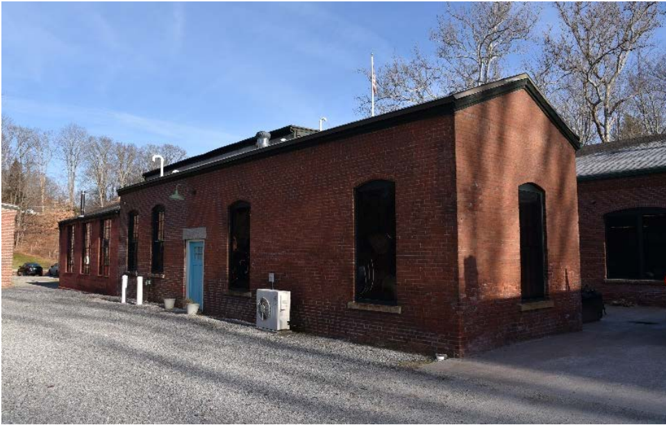
Photograph 47. West and south elevations of engine & boiler blocks with concrete block extension at far left; camera facing north/northeast. The architectural features of the boiler block distinguish it as a different construction date than the engine block.
