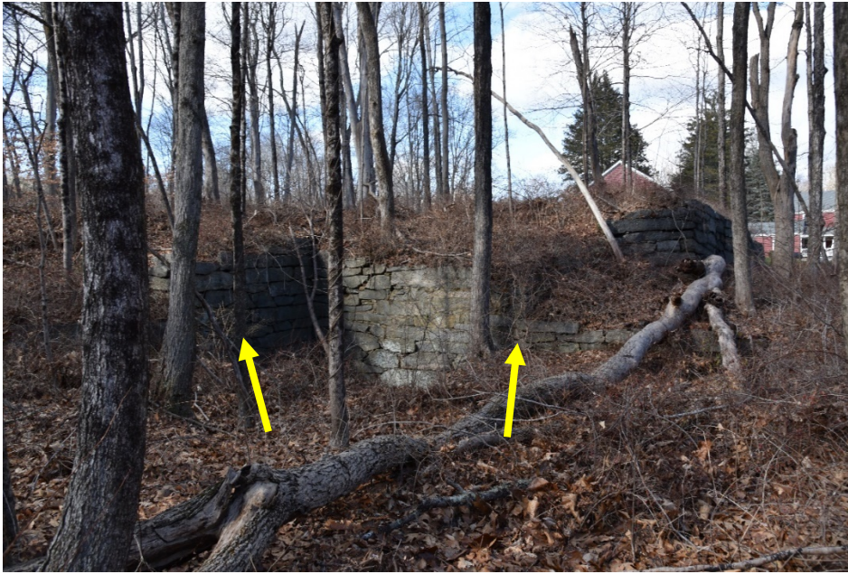
Photograph 6. Granite foundation walls of east/west forge at left and north/south forge at right; camera facing north.
