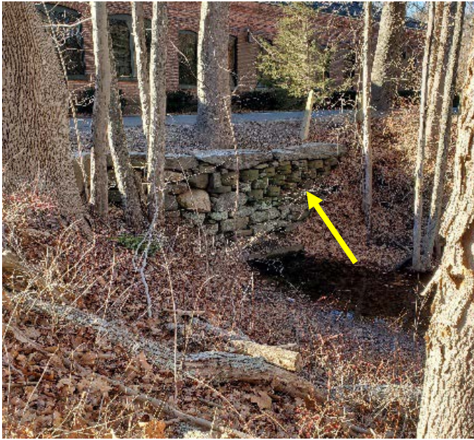
Photograph 41. After passing beneath the engine room, the tail race exits to the east, beneath Scovil Road north of the office, to rejoin the brook which runs along Candlewood Hill Road. A close look shows the bridge wall made partly of used grindstones.
