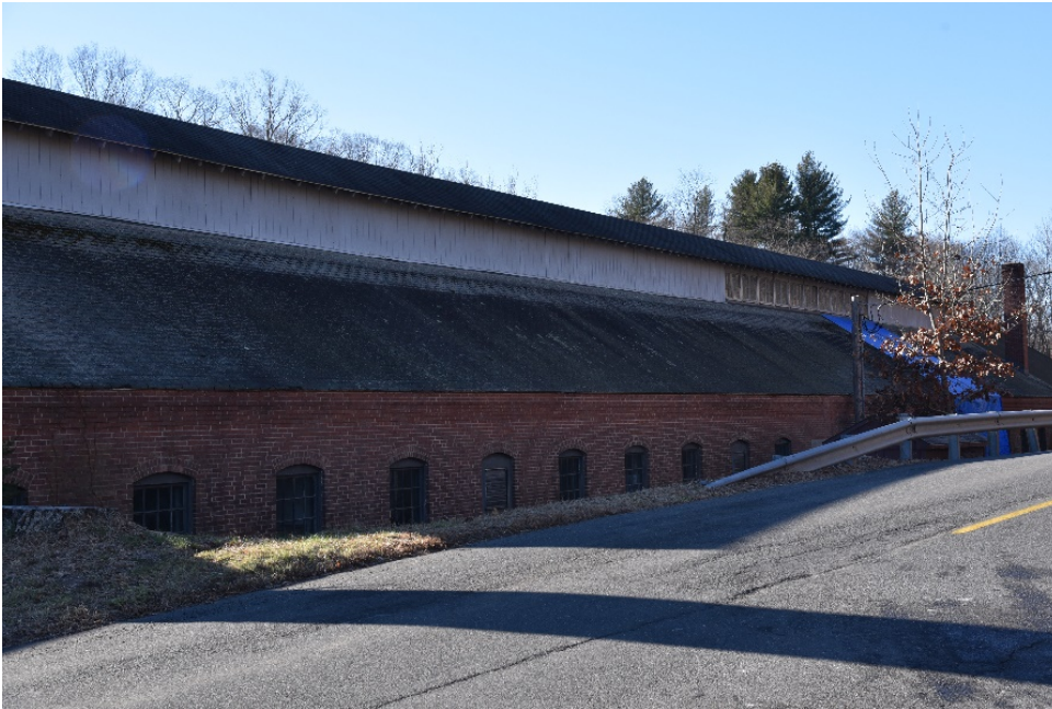
Photograph 96. North elevation of drop forge building; camera facing southwest. Openings on north wall, against Candlewood Hill Road embankment, have not been altered.
