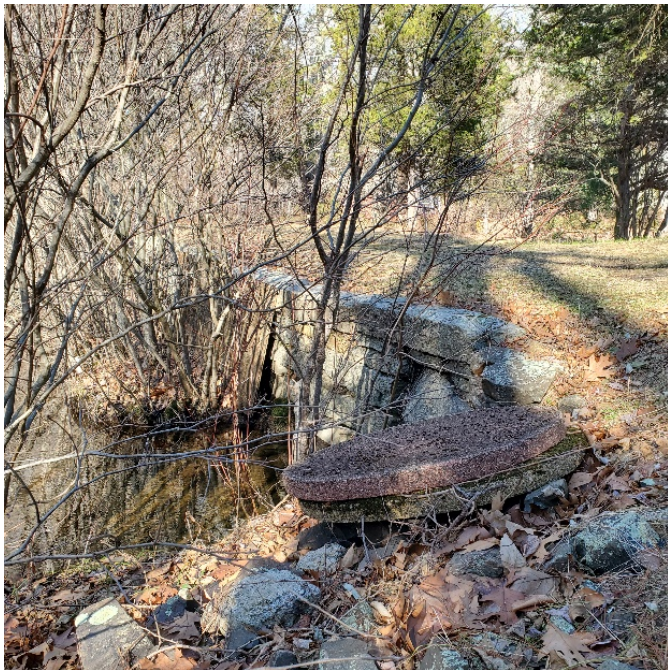
Photograph 12. Bridge over brook water where it connects with the pond; camera facing north.
