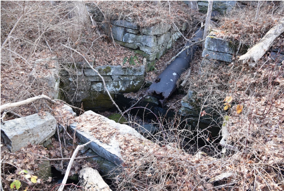
Photograph 5. Another flume discharge at the south end of the main forge ruins; camera facing west/southwest.
