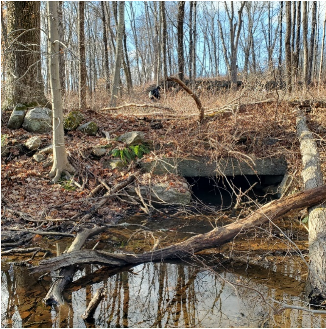
Photograph 11. Stone header for tailrace/brook beneath drive on east side of mill ruins in background; camera facing west.
