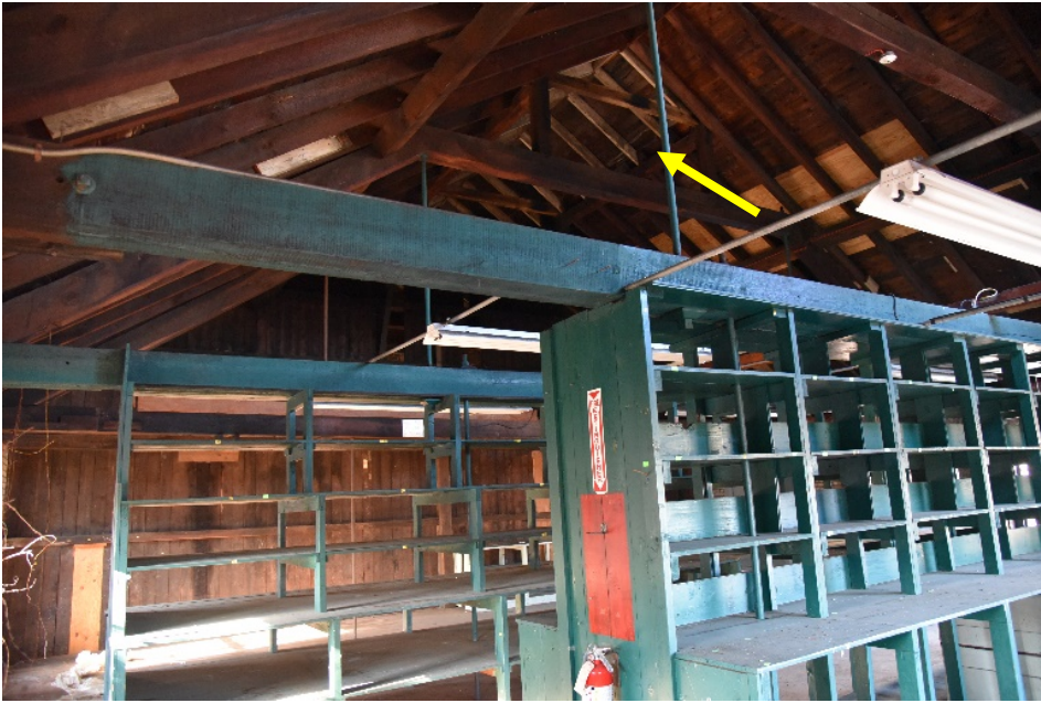
Photograph 94. Woodworking room looking toward firewall; section of newer roof framing at the ridge line is in place of former monitor.
