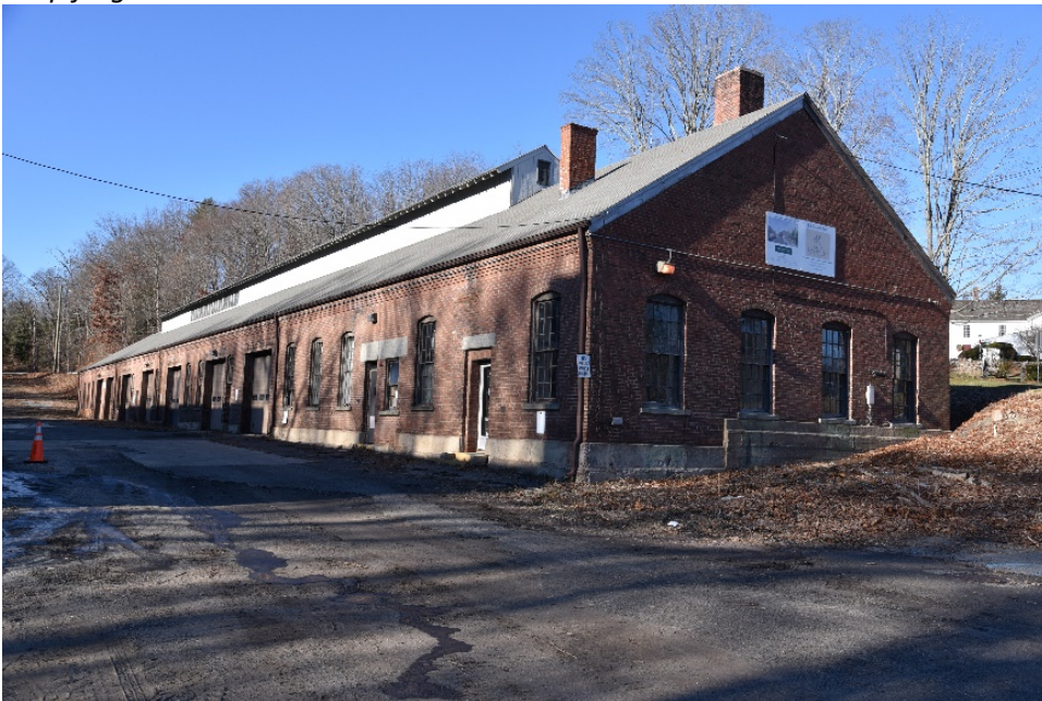
Photograph 95. South and east elevations of drop forge building; camera facing northwest. Fenestration on east wall is unchanged.
