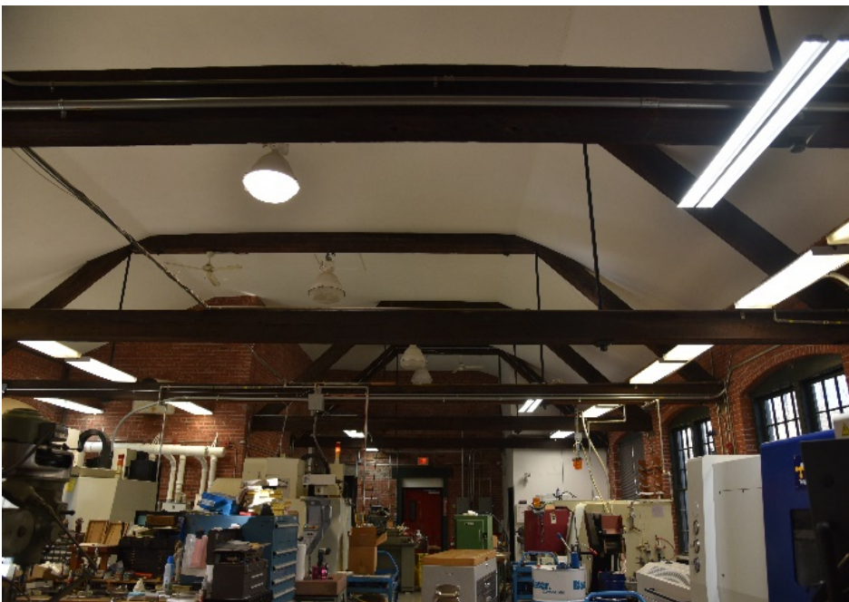
Photograph 53. Interior of polish room with partially exposed truss framing and east end of engine block in left background; camera facing north. The framing is built into the engine wall at the far end indicating its construction or expansion postdates the engine block.
