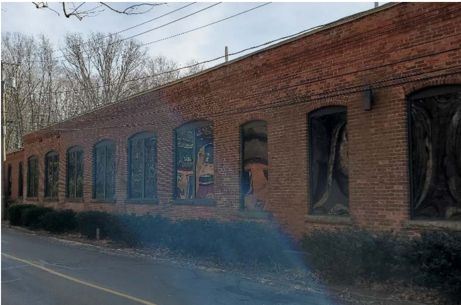
Photograph 49. East elevation of grinding/forge room (R) where it joins the polish room (L); camera facing south.
