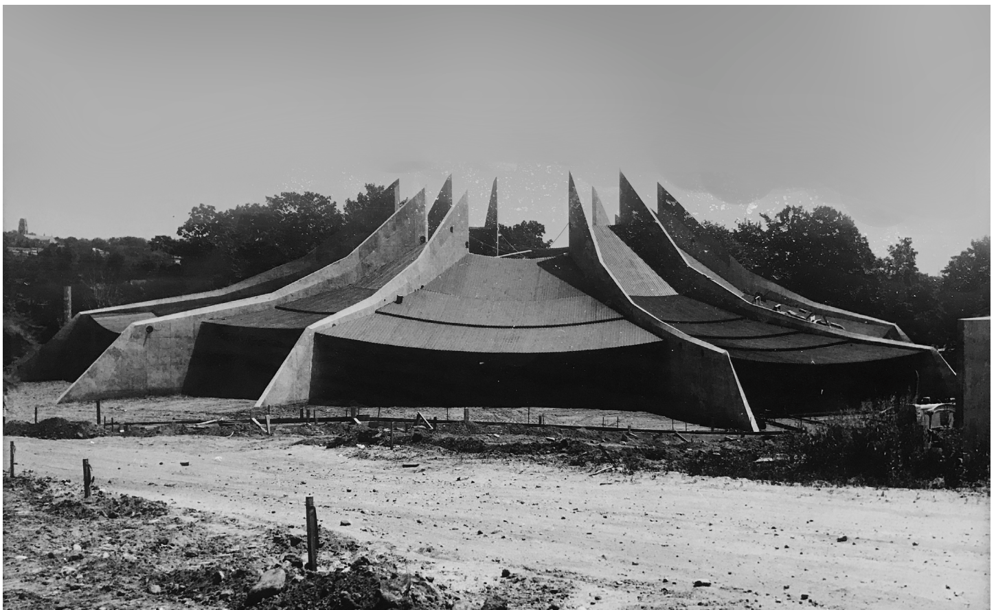
Figure 3 of 13. Construction progress, showing the completion of the roof cables and wood decking, June 1, 1964. Archives of the Unitarian Society of Hartford.
