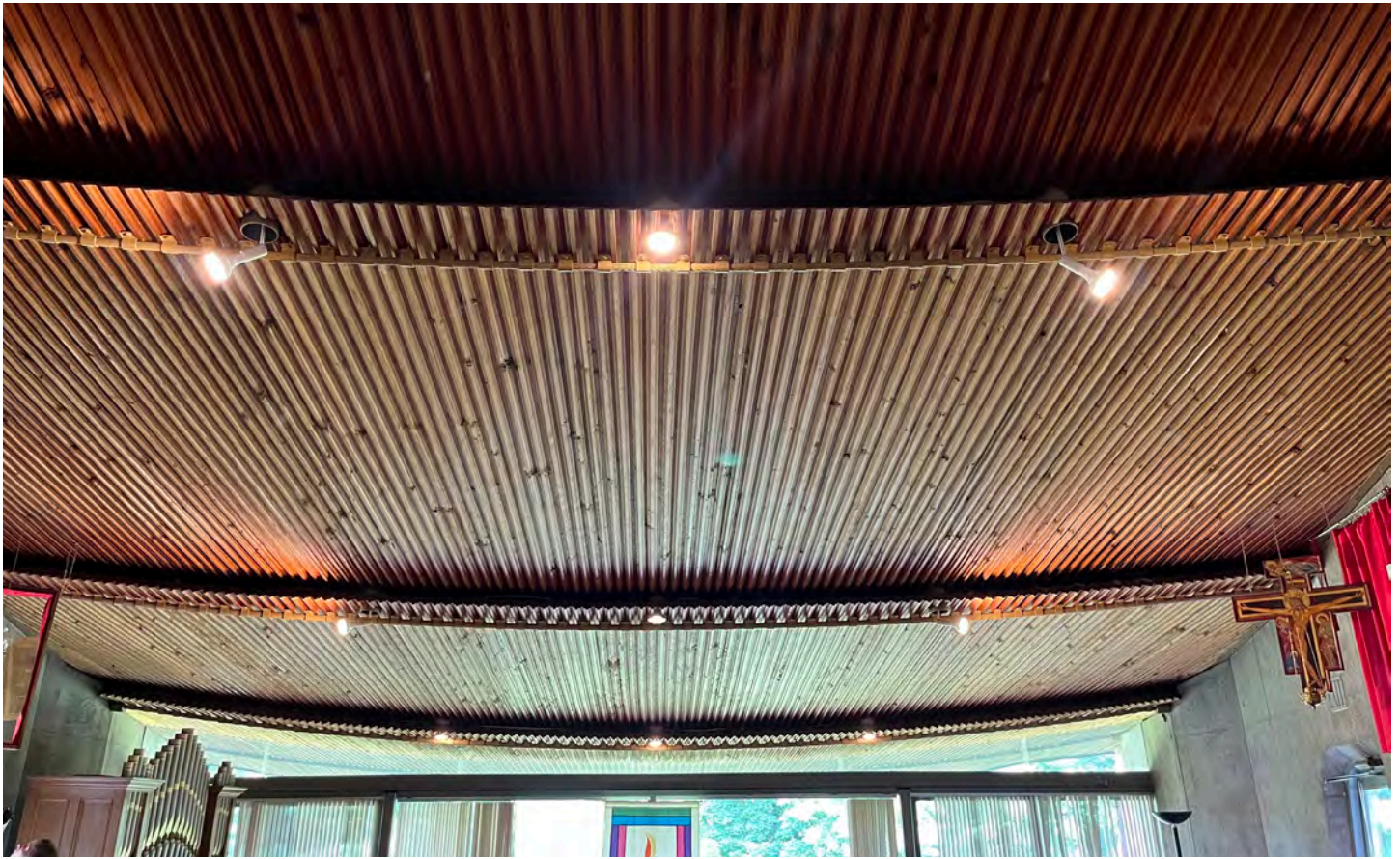
Photograph 19 of 29. Detail of the exposed underside of the roof's wood decking as seen from the chapel.
