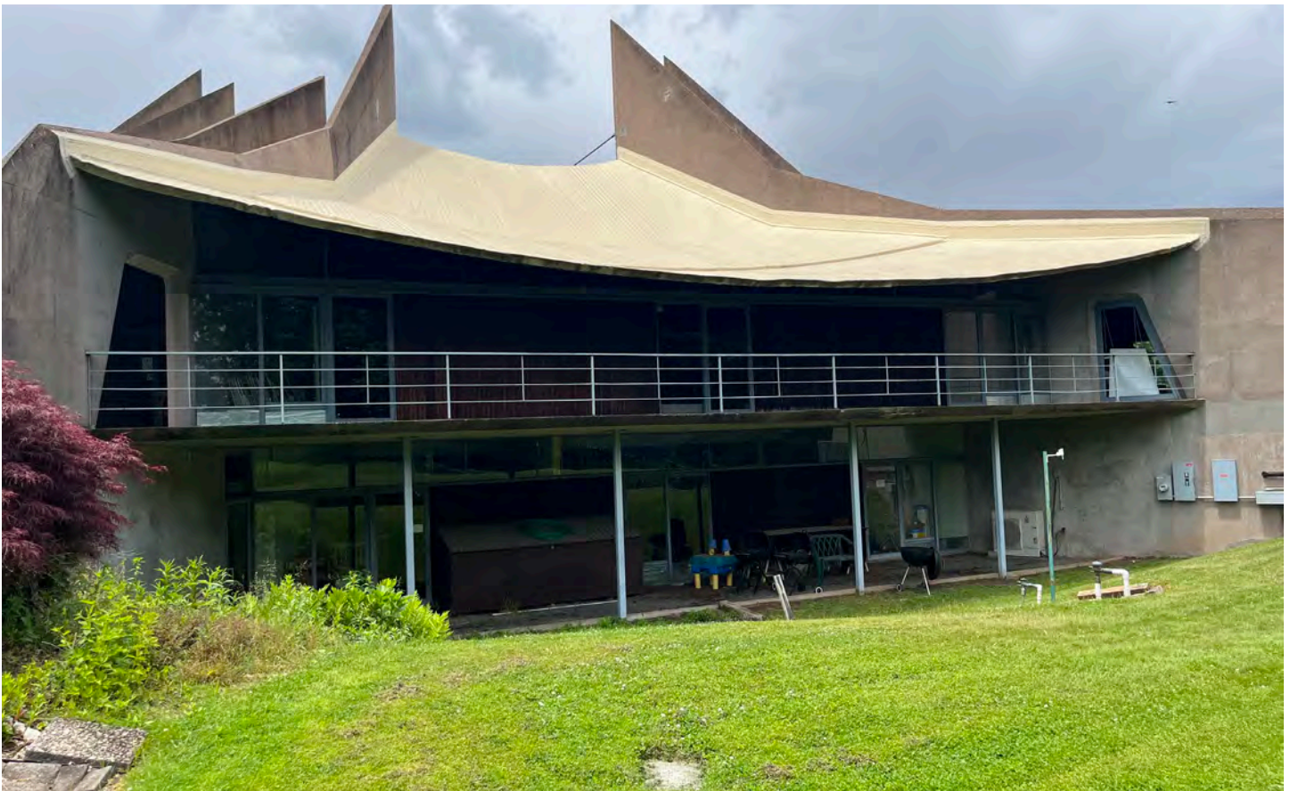
Photograph 10 of 29. Easternmost bays showing the exterior balconies at the main level and the sunken courtyards at the basement level.
