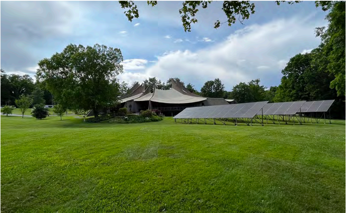
Photograph 3 of 29. Photovoltaic panels at the southwest corner of the property.
