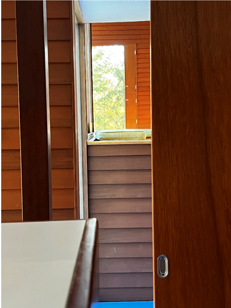
13 of 21. Sliding panel door in kitchen, looking south towards conversation pit and living room. Level 3.
