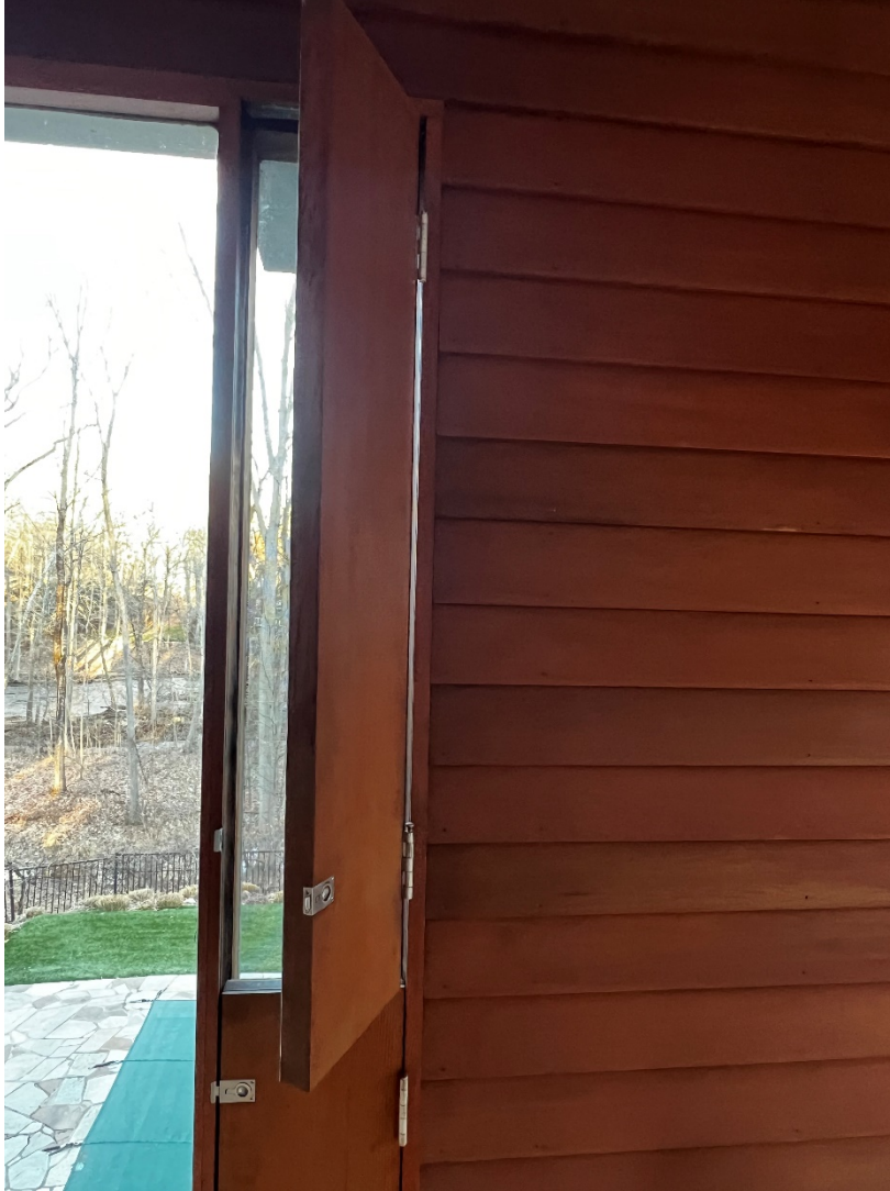
18 of 21. Detail of ventilation panels in living room, looking south. Level 4.
