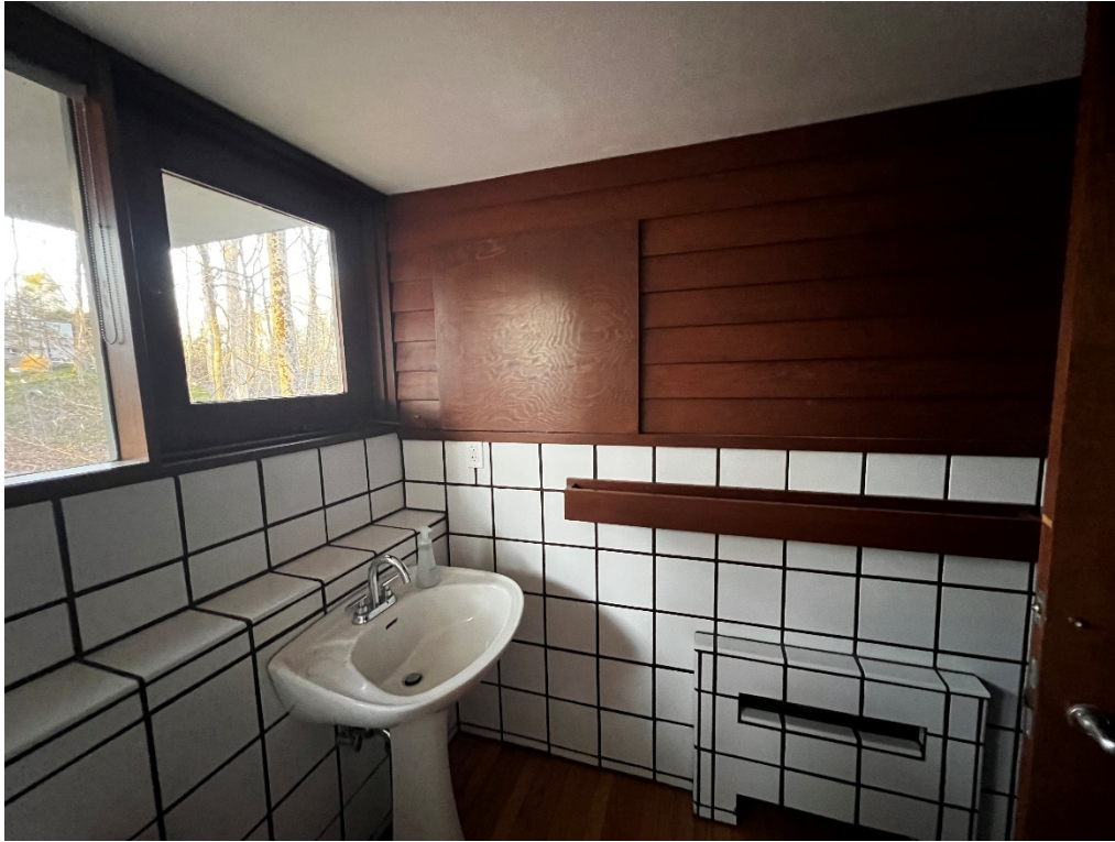
10 of 21. Detail showing original remaining cedar paneling, windows and built-in medicine cabinet with mirror in bathroom, looking north. Level 1.
