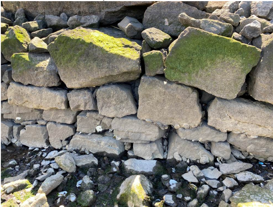
Figure 12. Detail of Long Wharf Pier structure, looking southwest (2021, New Haven Preservation Trust).
