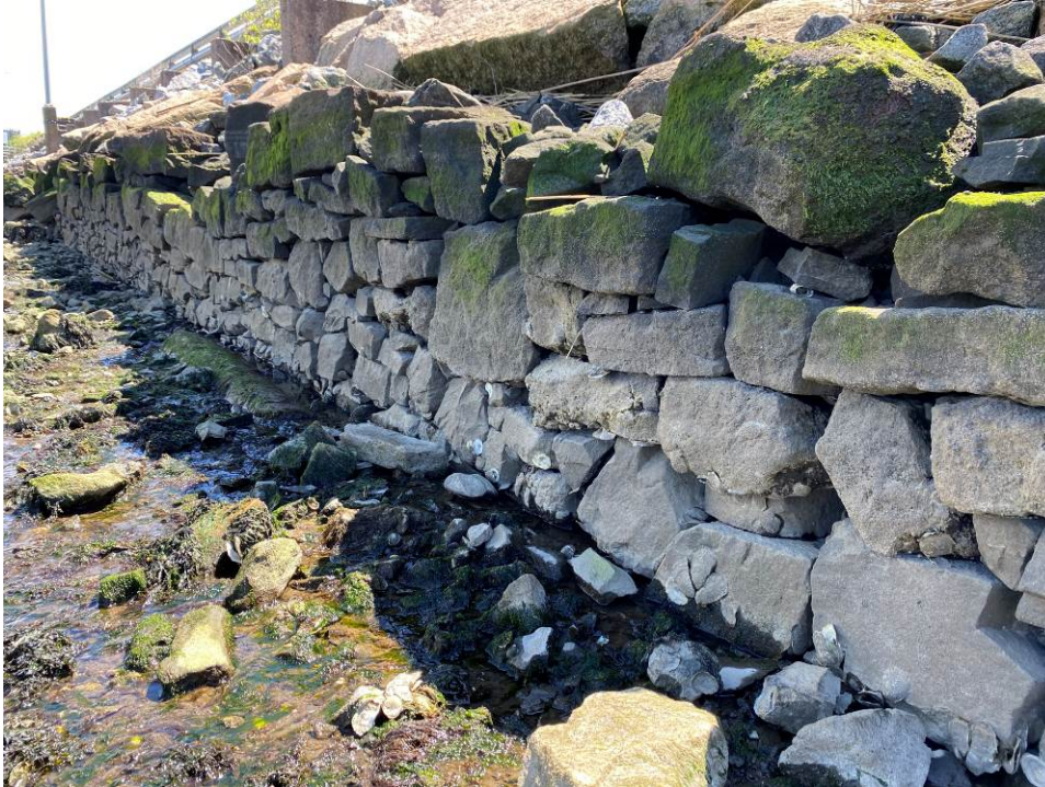
Figure 11. Long Wharf Pier structure, showing stone walls laid by Lanson (2021, New Haven Preservation Trust).
