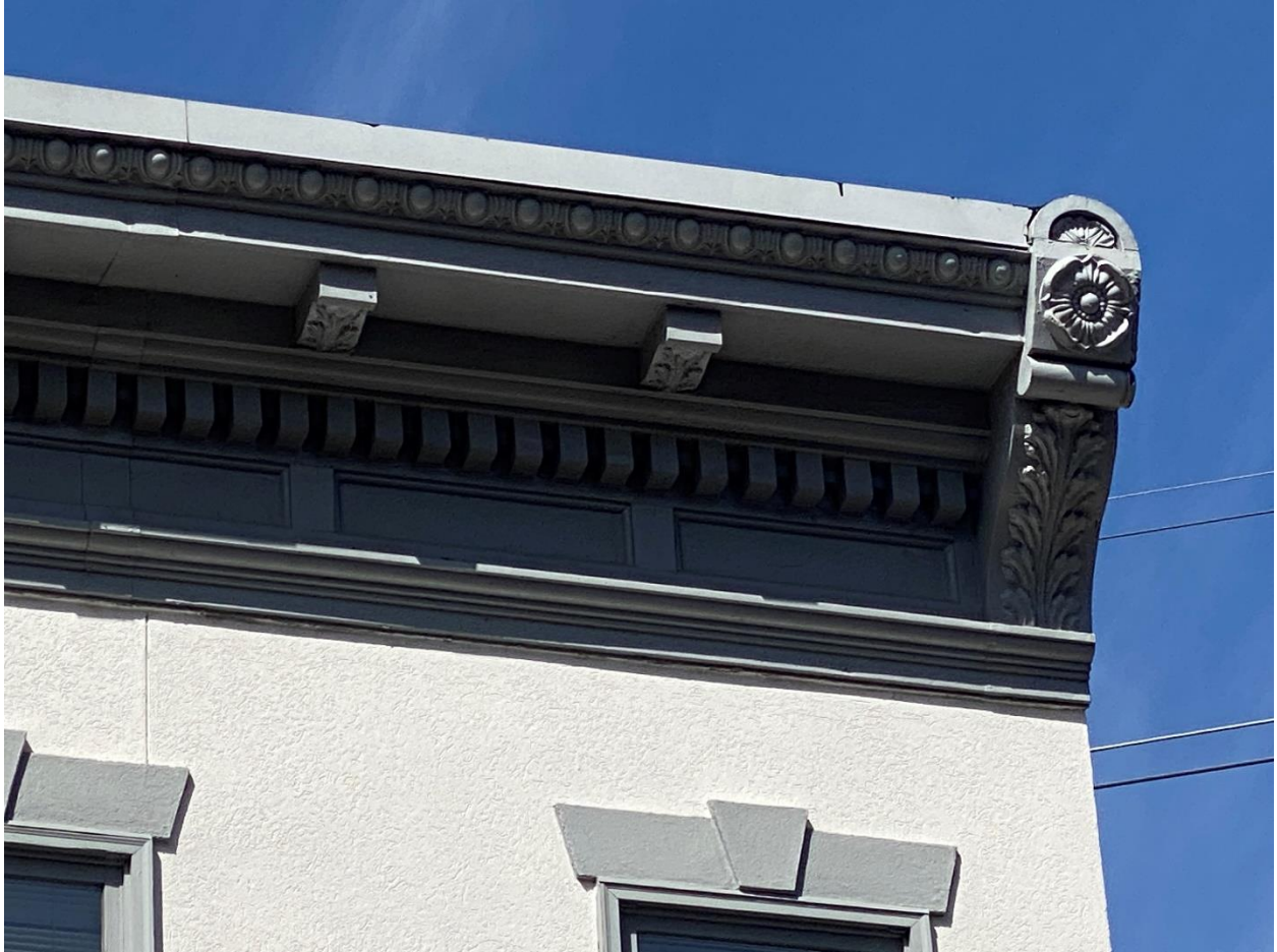
Photo 3 The sheet metal cornice is intact and is the only remaining original feature of the façade.
