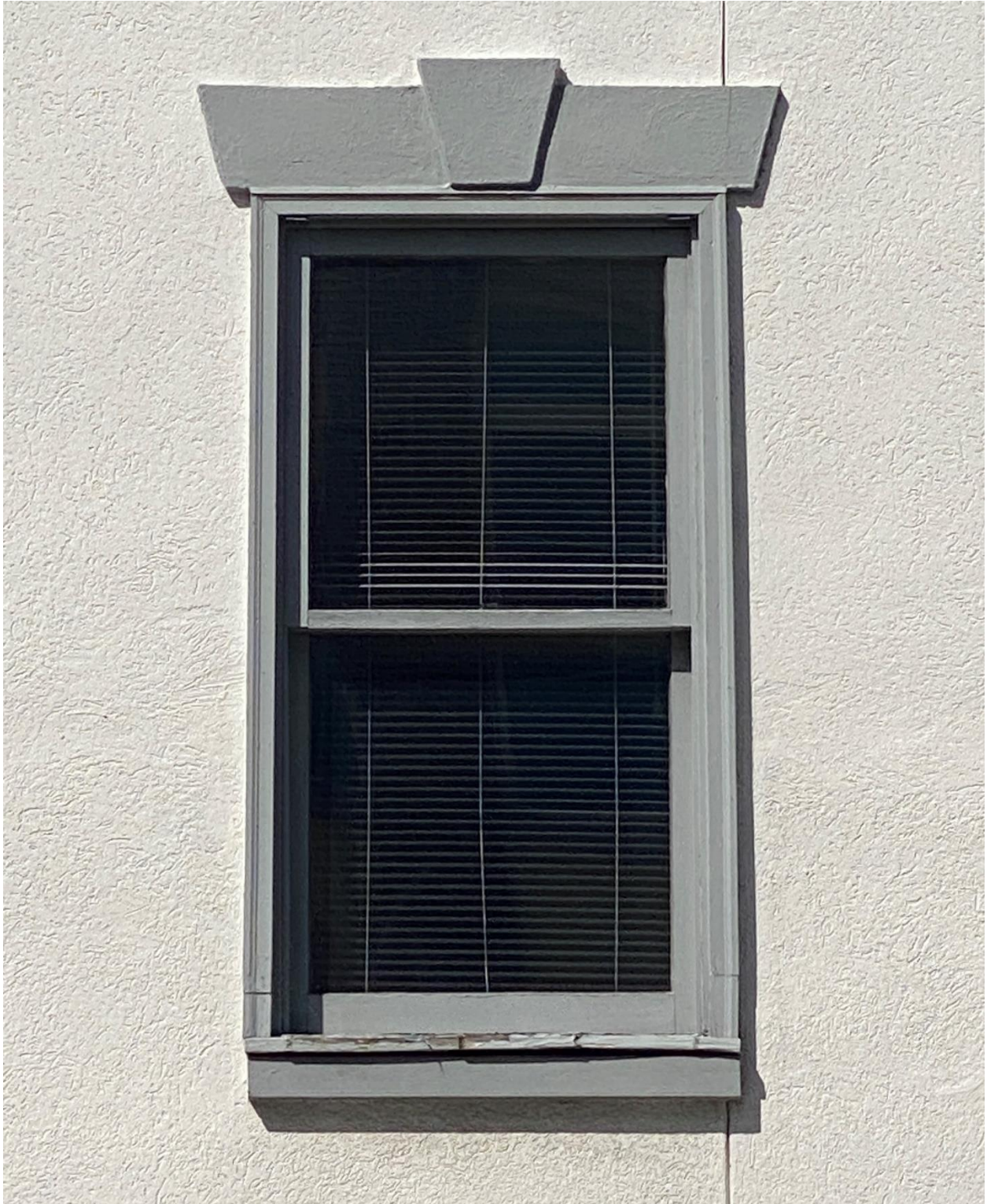
Photo 4 New windows were fabricated of inferior materials, and are deteriorating. Original flat sills and lintels have been altered in an unfortunate manner. The exterior aprons are of dimensional lumber.
