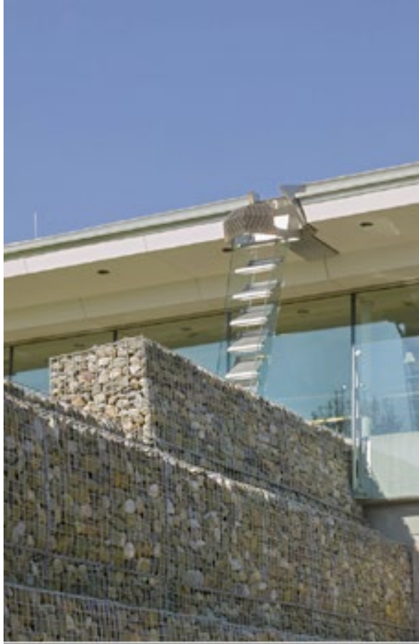
Photograph 10. View of retaining wall and roof detail on east elevation, facing southwest.
