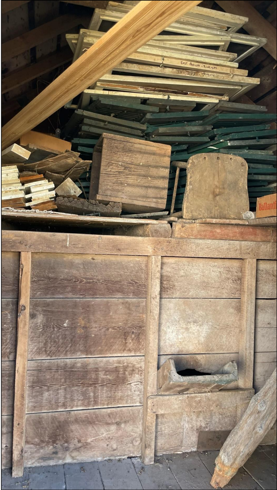
Photograph 22 – Looking east in the western section of the granary. The chute connecting the two spaces is visible in the lower right corner. (5387)
