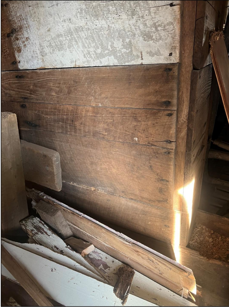
Photograph 15 – Looking east at one of the insulated walls in the west end of the west barn. Circular saw marks are clearly visible on the boards, which are fastened with wire nails, while sawdust infill can be seen on the right where a board has been removed from the bottom of an opening in the wall.
