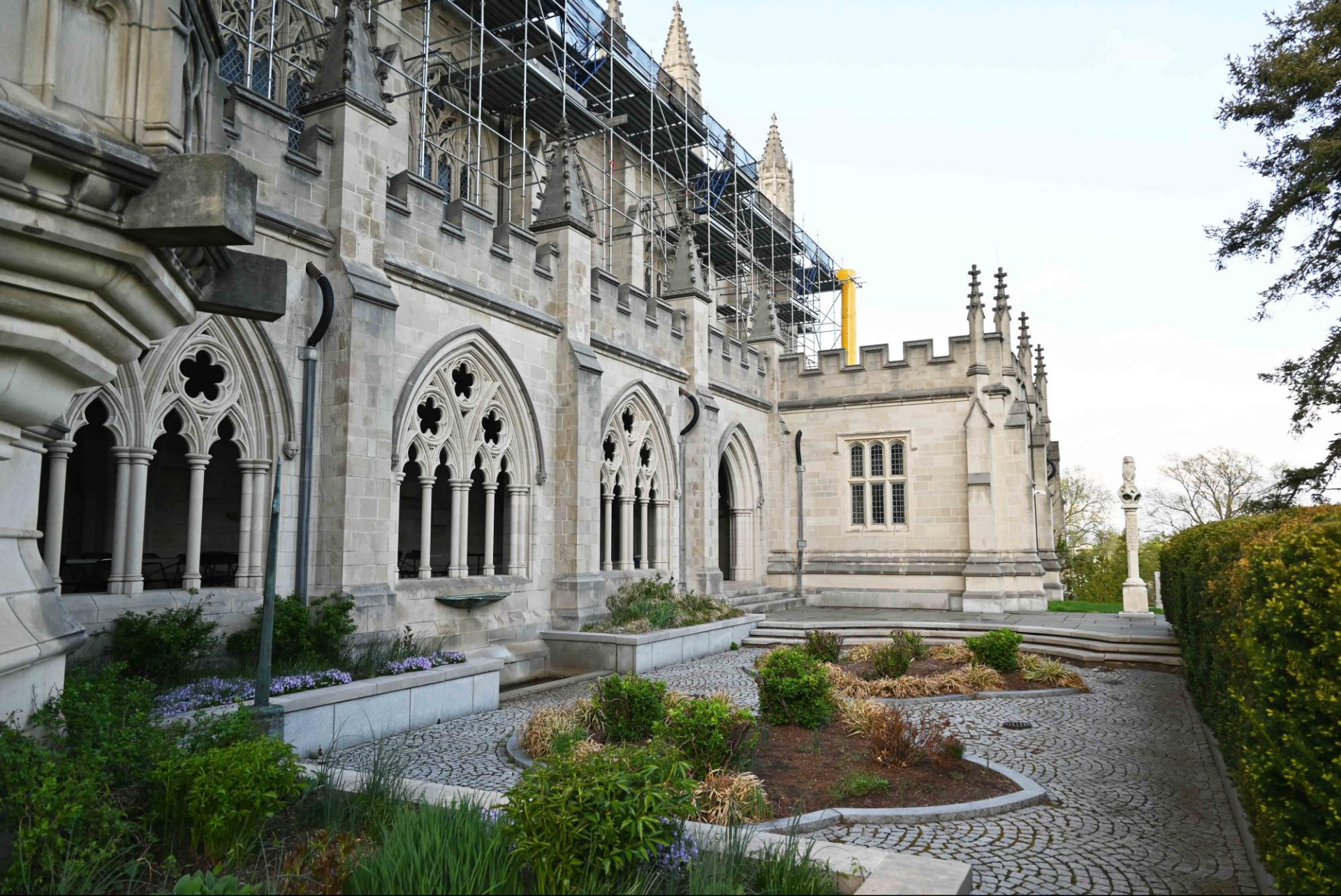
Chapel's south cloister, south wing, and garden, camera facing east. Trinity College Long Walk Historic District Hartford County, Connecticut
