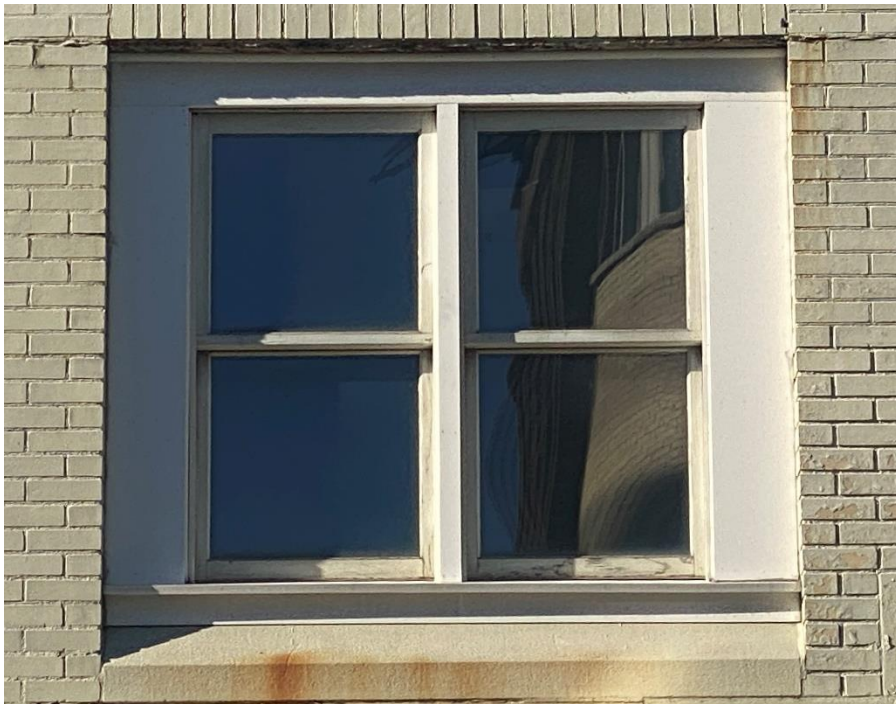
Photo 6 Windows on the building are inappropriate and will require appropriate replacement.
