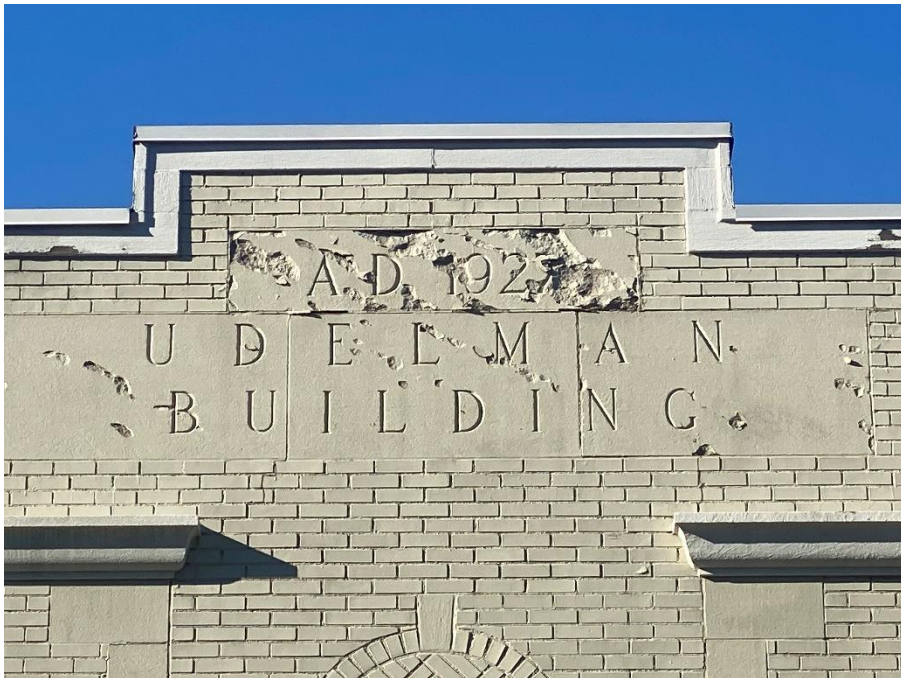
Photo 4 Limestone spalling will require significant intervention affecting building integrity
