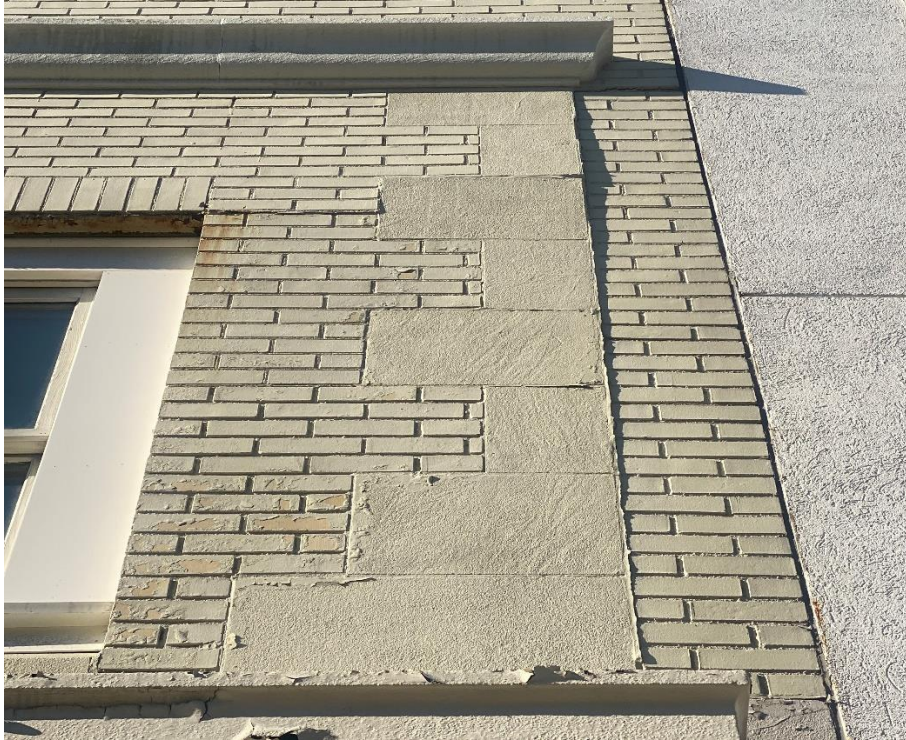
Photo 3 Stone masonry has been seriously displaced and presents a hazardous condition
