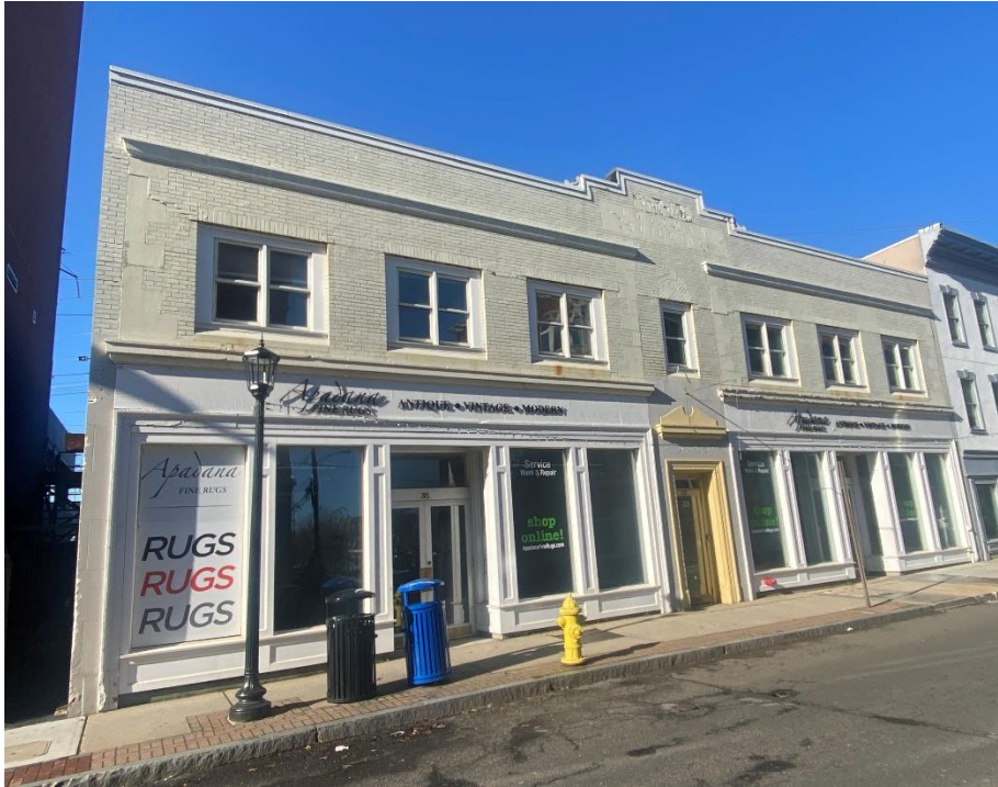
Photo 1 Paint obscures much of the damage and deterioration on the building façade
