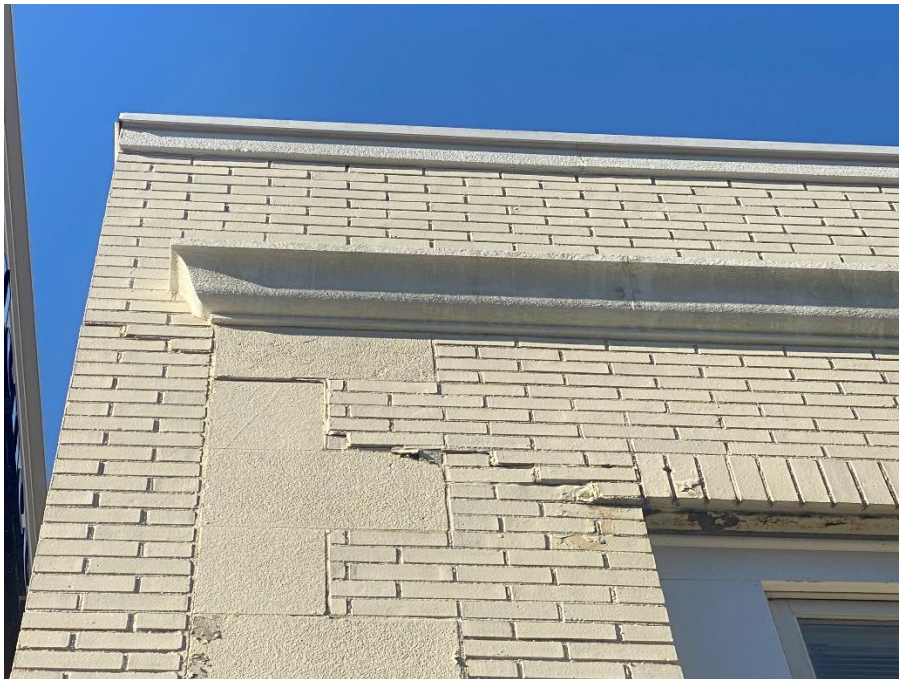
Photo 2 Oxide jacking of steel has resulted in serious damage to brick and stone masonry.
