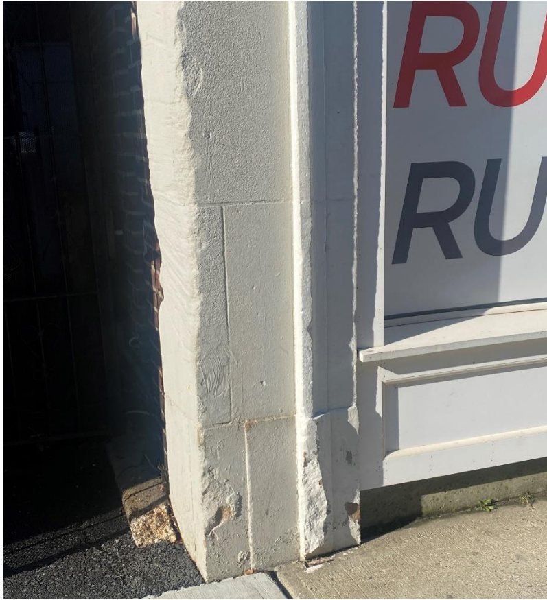
Photo 5 Ashlar quoins at the building ends are damaged and unsightly
