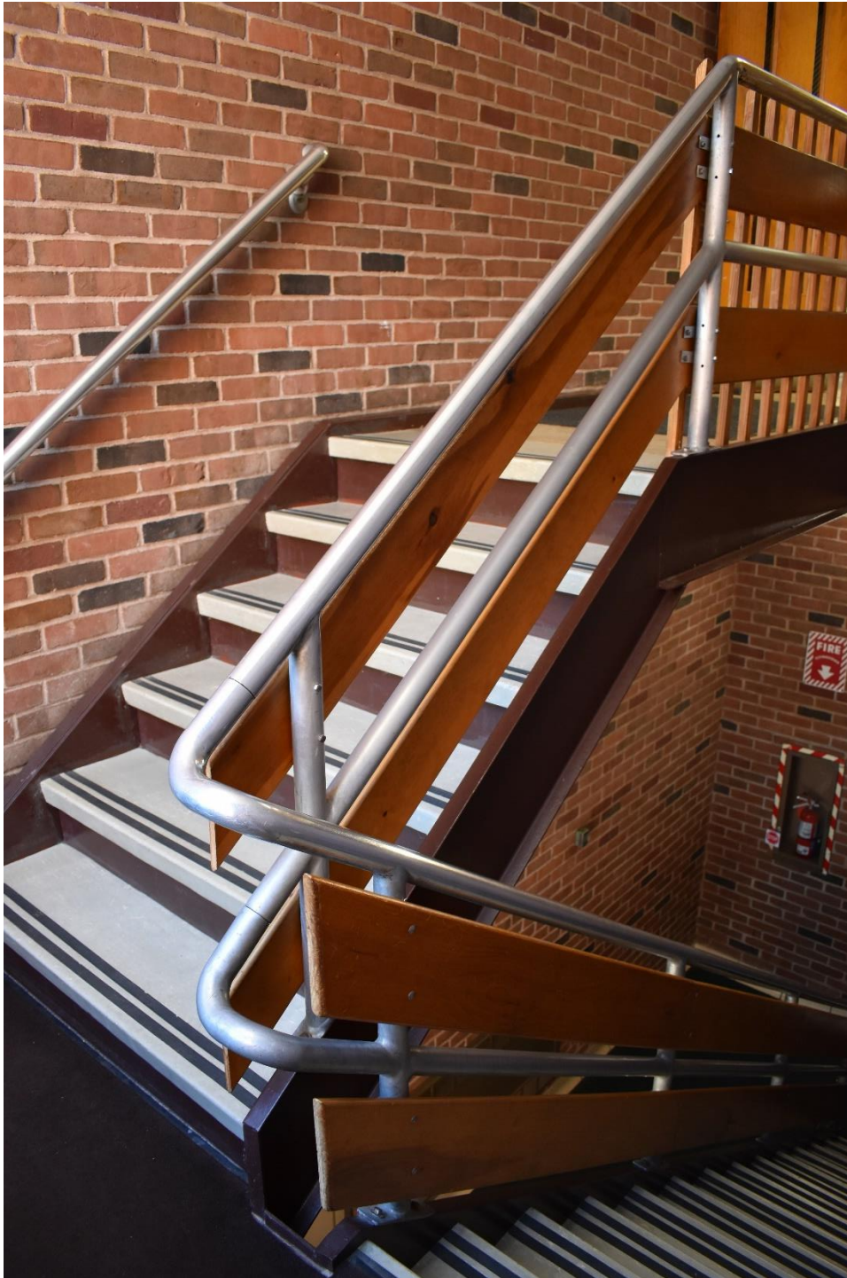
Photograph 42 of 42. Typical stairwell in the 1972 addition to the building. Camera facing southwest.
