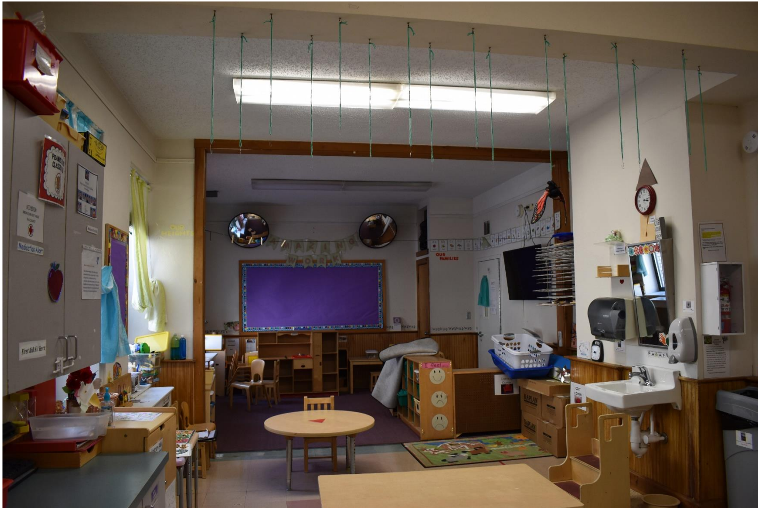
Photograph 18 of 42. Typical classroom in the 1928 section of the building. Camera facing east.
