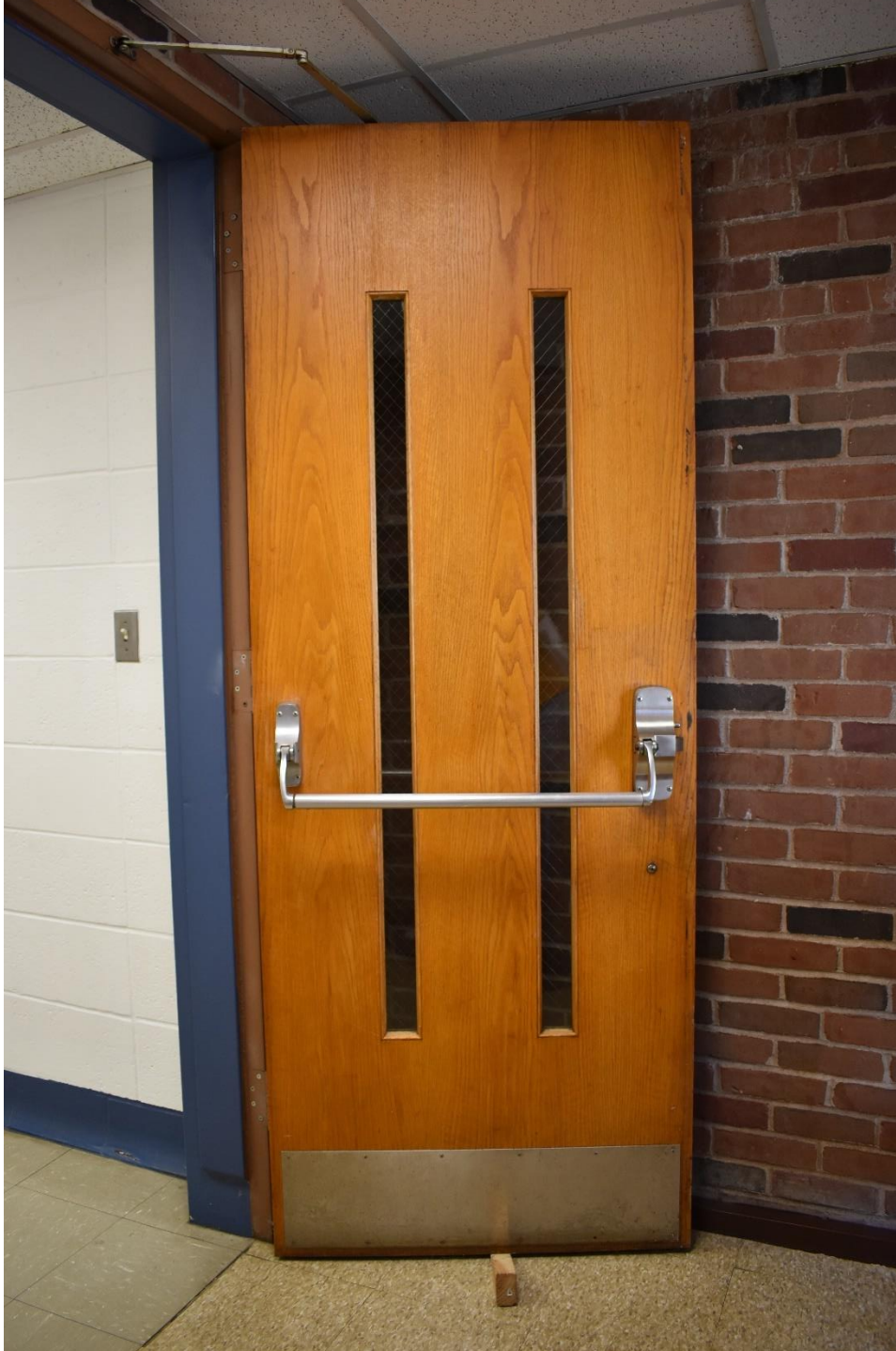
Photograph 41 of 42. Typical hallway door in the 1972 addition to the building. Camera facing northeast.
