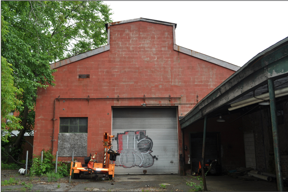
29. Stanley Rockwell Company Factory, west and north elevations 1966 and 1962 loading dock, camera facing east.
