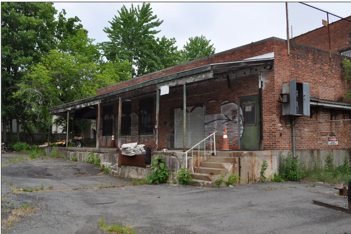
32. Stanley Rockwell Company Factory, west and south elevations 1962 loading dock and 1944/46 shipping and storage block, camera facing northeast.
