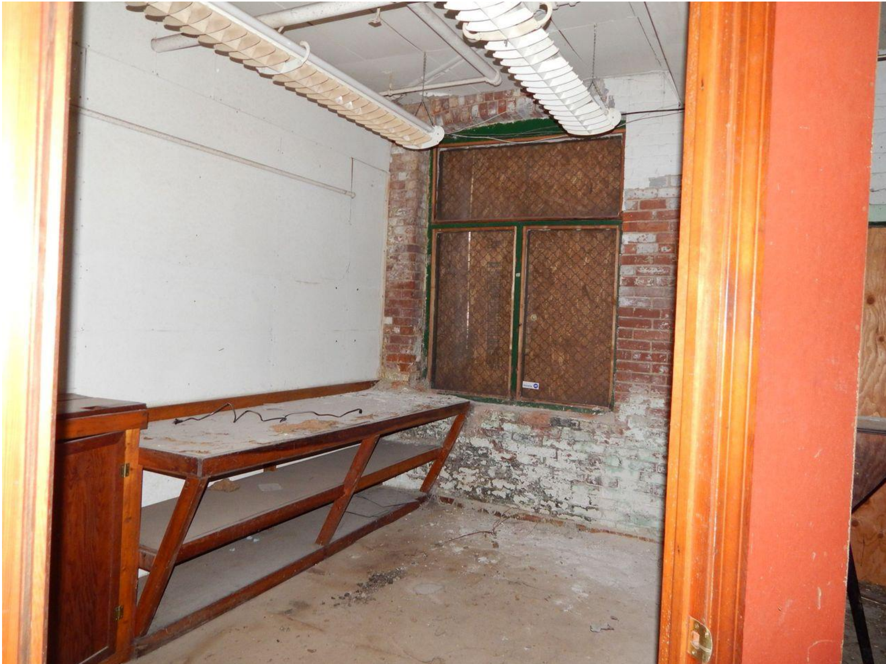
First floor interior storage room along western wall. Camera facing west. Photograph 13 of 37
