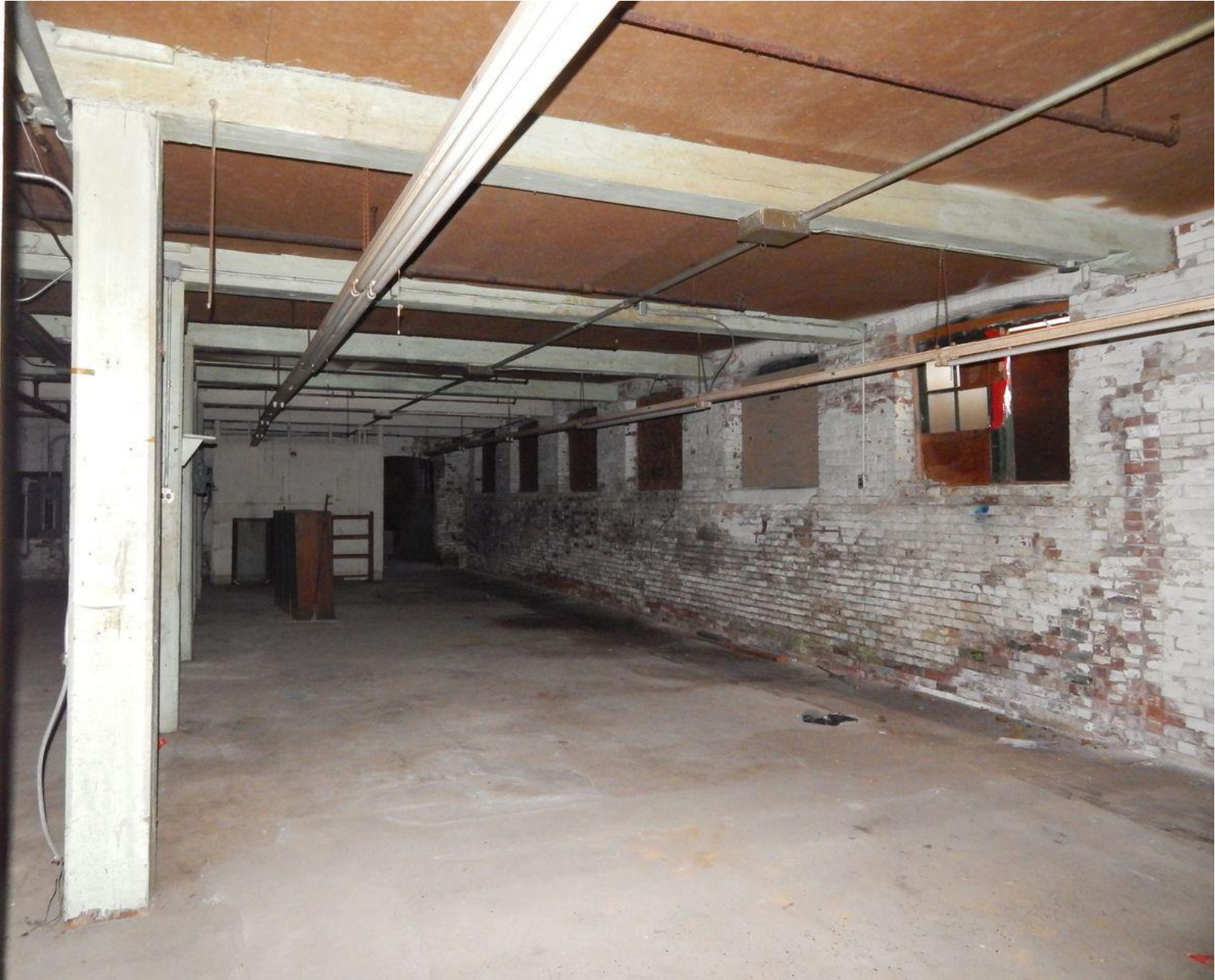
First floor interior space. Camera facing north from center of room Photograph 16 of 37
