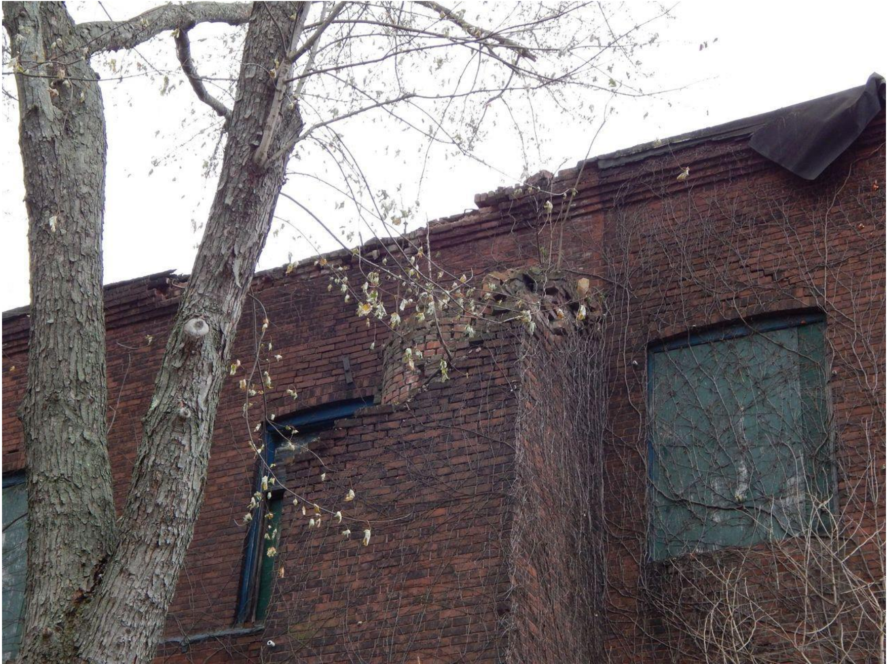
Detail of enclosed smokestack along northern elevation. Camera facing south. Photograph 10 of 37
