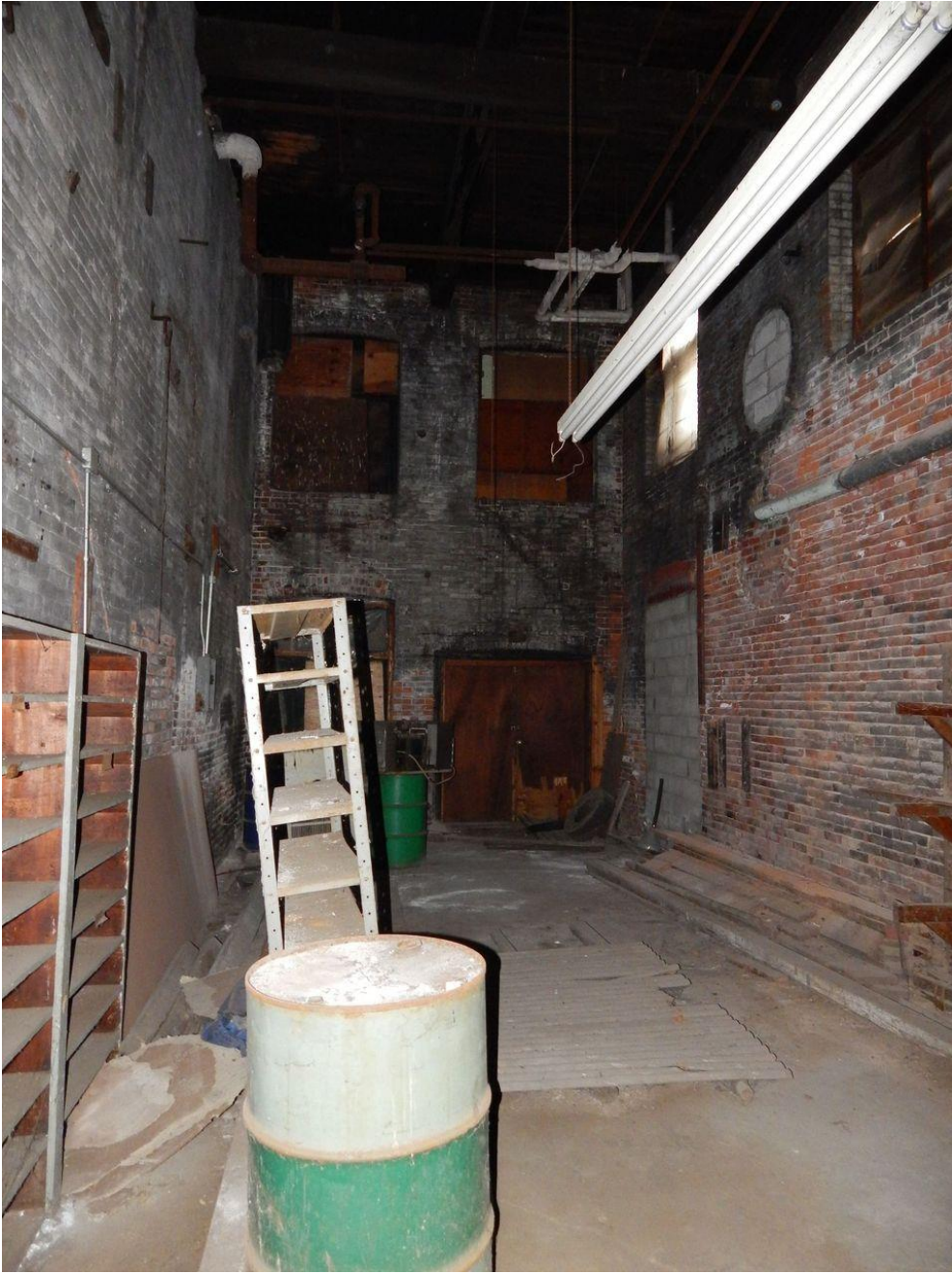
Interior of northern boiler room. Camera facing west.
