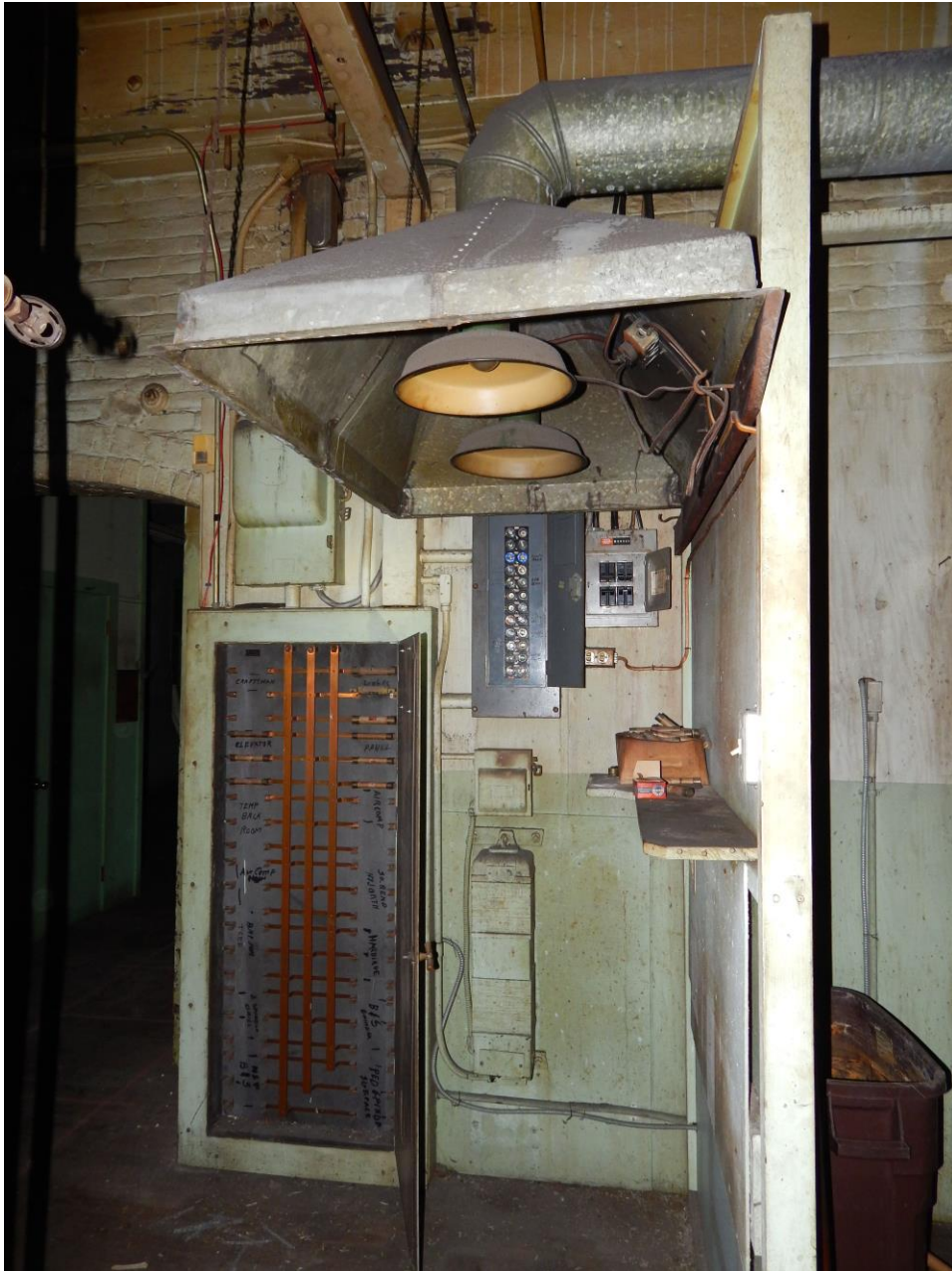
Second floor fuse panel and electrical service. Camera facing north. Photograph 30 of 37
