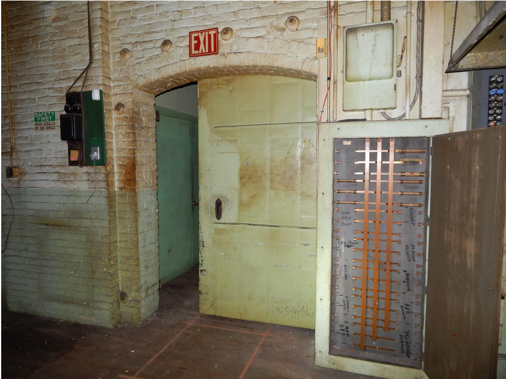
Second floor. Automatic fire door (seen throughout). Camera facing north. Photograph 28 of 37
