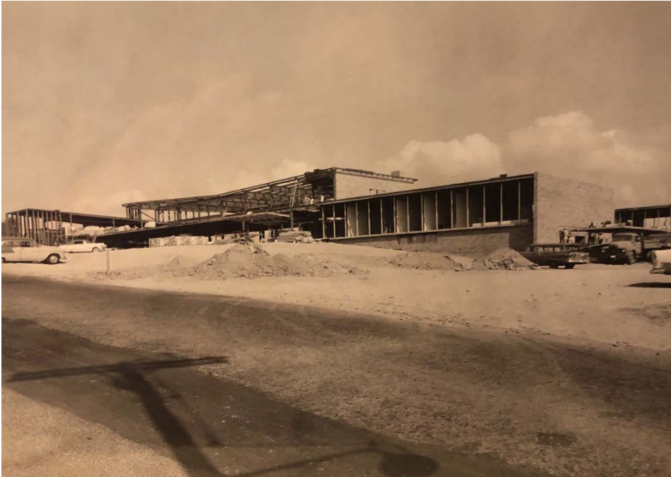
Figure 8 Construction, c. 1959. Camera facing northeast from Ridge Road. Notice curvature of roofline. Compare to Figure 4 and Photographs 7-8.
