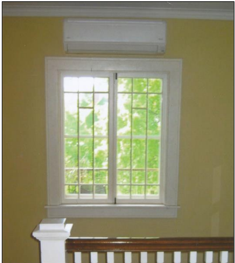
Ductless Mini-Split Unit. Source: Wisconsin History.
