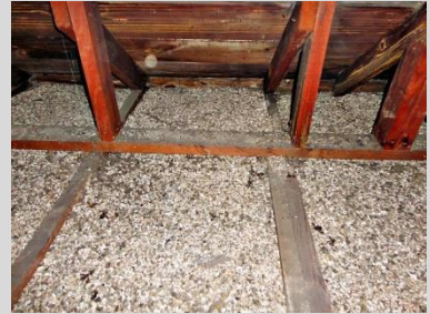
Vermiculite attic insulation. Source: Greenbuildingadvisor.com.
