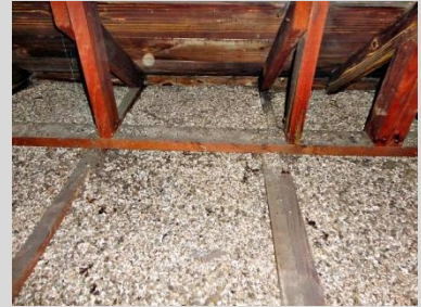
Vermiculite attic insulation. Source: Greenbuildingadvisor.com.
