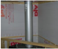
Manufactured fireplace installed with air barrier (gypsum board, Thermoply, or equivalent) in place. All seams caulked, taped, or sealed with expansive foam.
