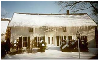
...Unenforced/ Badly Detailed Energy Code Requirements!!! - Second Highest Insurance Claim In NY
