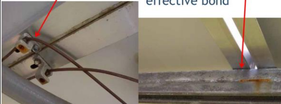
Aluminum bolted to steel without isolation washers and no effective bond
