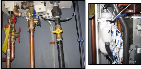
Noritz tankless with condensate neutralizer with No Recirculating line. 88
