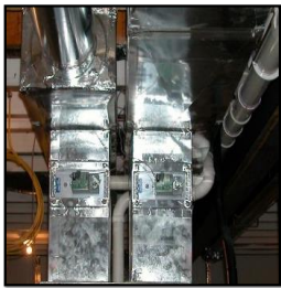
First and second floor zone dampers
