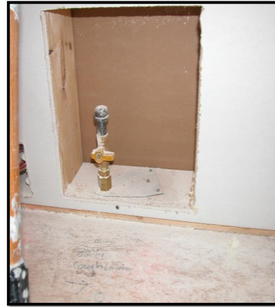
Gas outlet for kitchen range
