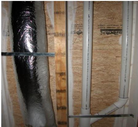
Looking up at basement ceiling, flex duct and furnace venting
