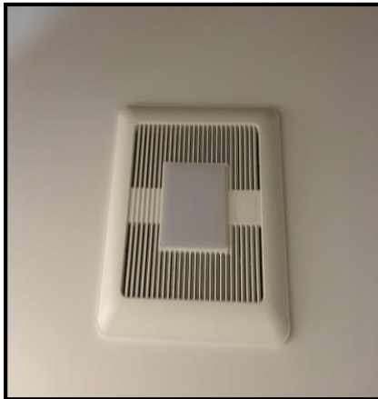
Bath exhaust used as part of ventilation system
