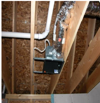
1 of 2 exhaust fans with programmable CFM exhaust 114
