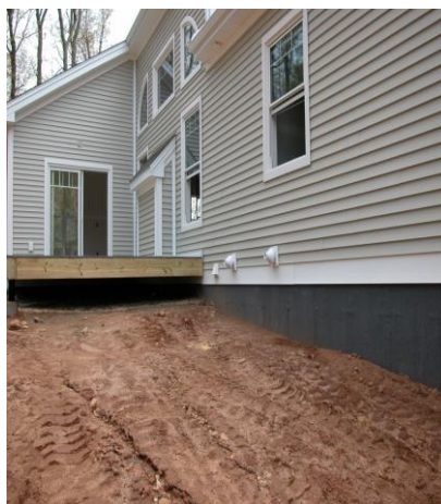
Dryer, Water heater, Furnace vents
