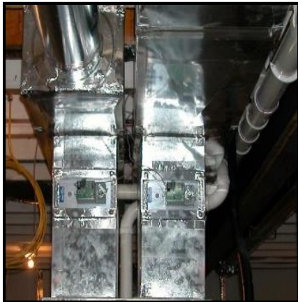
First and second floor zone dampers
