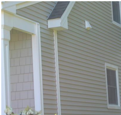
Exhaust opening for Range hood
