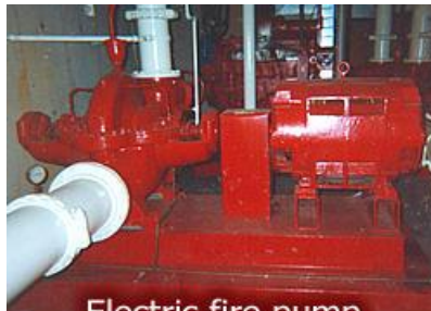
Electric fire pump
