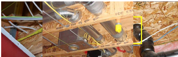
Multiple penetrations near support
