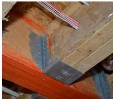
Hanger Does Not Restrain Top Flange ➤ Web Stiffener Required
