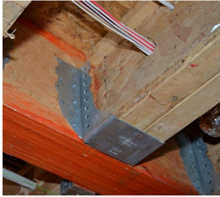
Hanger Does Not Restrain Top Flange ➤ Web Stiffener Required
