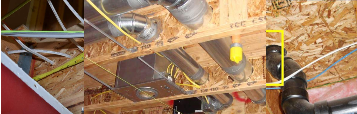
Multiple penetrations near support
