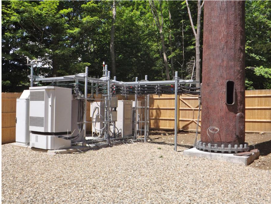
AT&T equipment pad
