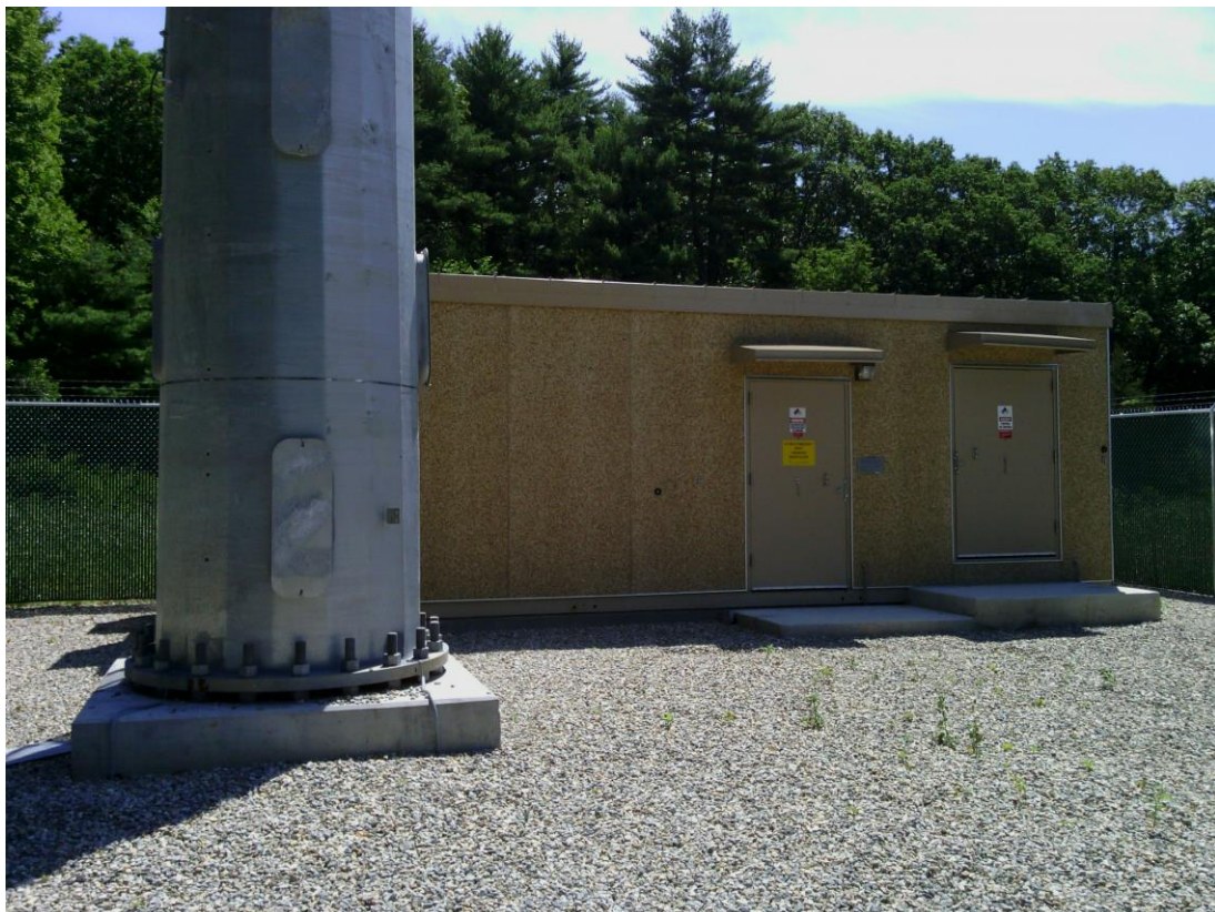
Interior compound view. Fuel tank behind shelter.
