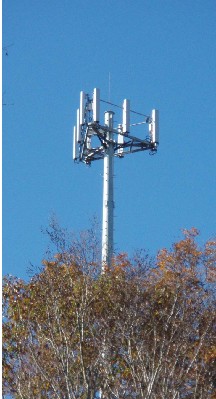
Close up of antennas mounted at top of tower
