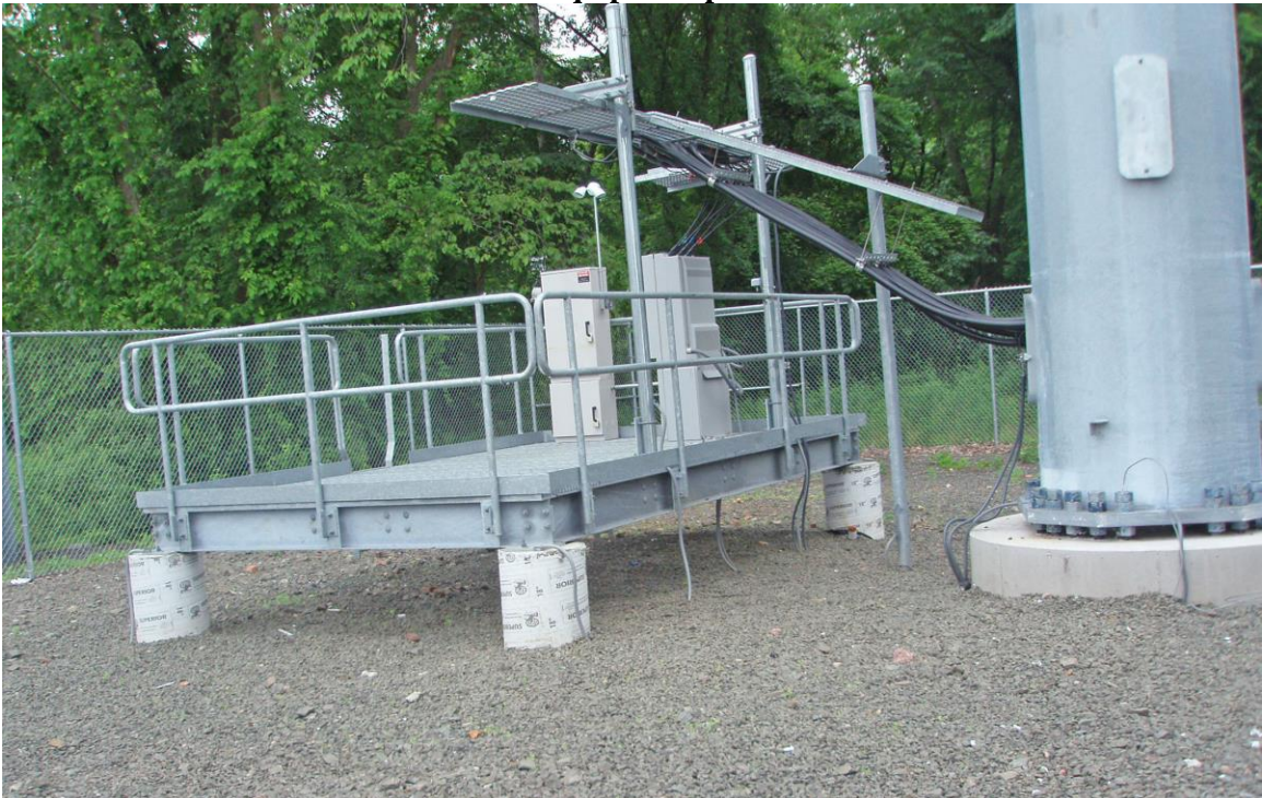
View of equipment platform
