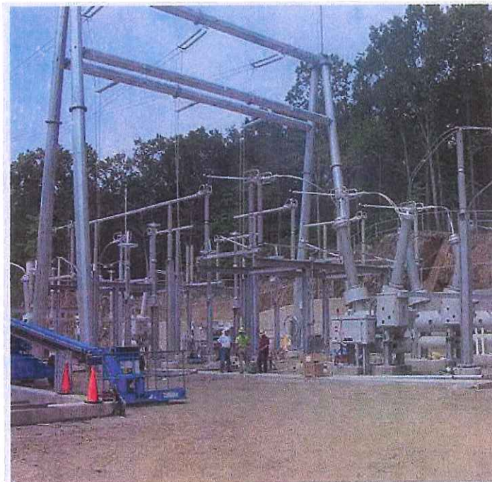
Figure C-1: Archers Lane 345-kV Transition Station
