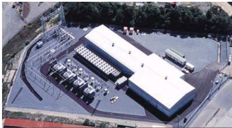
Figure 24 The 330 MW Cross Sound Cable converter station at Shoreham, L.I.
