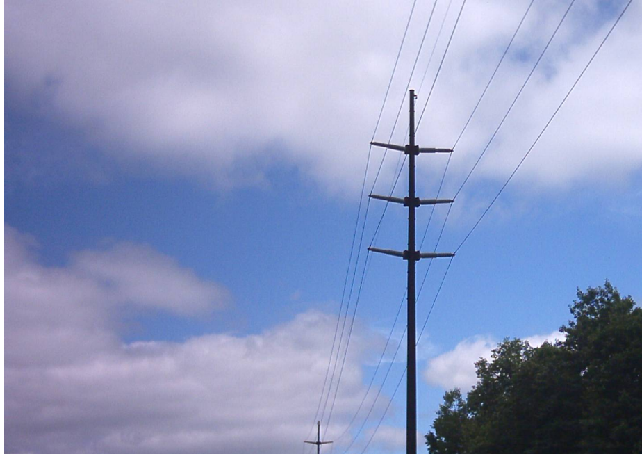
Figure 5. Split-phase line with reverse phasing near Sidney, NY. The split-phase line is adjacent to a railroad.
