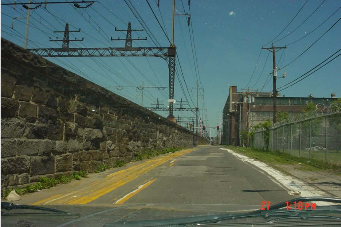
Photo 8. Railroad Avenue (EB) looking eastbound toward the Howard Avenue intersection. Note the poor pavement condition.
